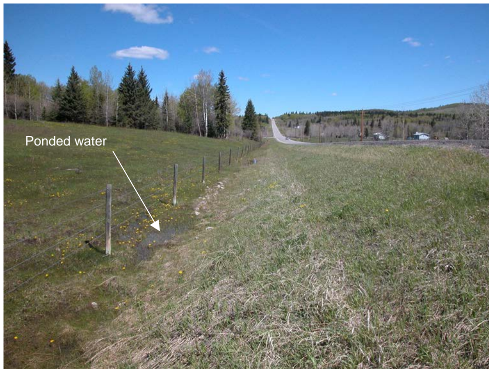
Photo S10C-3 (lower left) – May 2004 – facing north along the west ditch downslope of the highway. Note the ponded water in the ditch. It appeared that the ponding of the water was due to the lack of ditch gradient through this area as well as groundwater seepage discharging from the toe of the slope.
