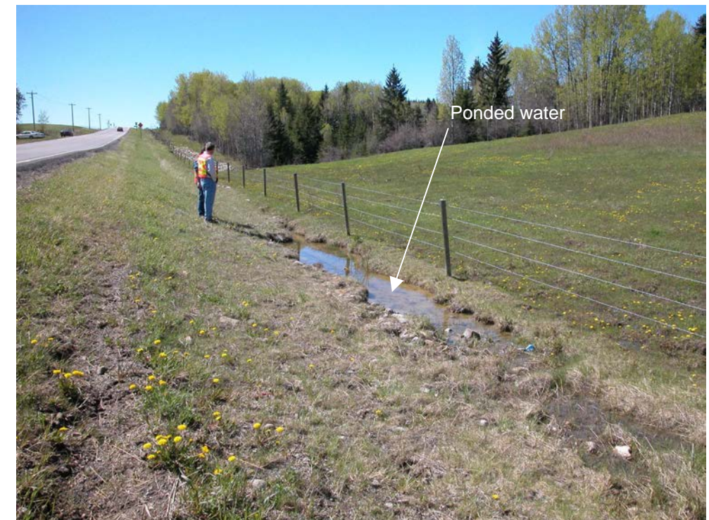
Photo S10C-4 (lower right) – May 2004 – facing south along the west ditch below the highway. It is recommended that a weeping tile drain be installed in this ditch to pick up accumulated surface runoff and groundwater seepage from this area. The weeping tile should drain to the south.
