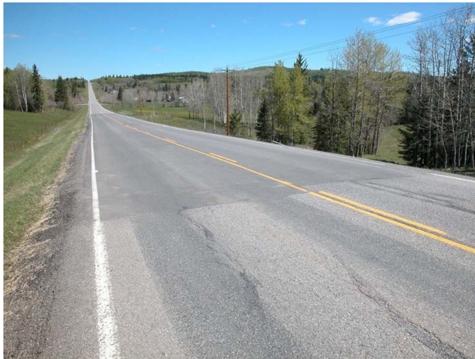
Photo S10C-1 (upper left) – May 2004 – facing north across the July 2003 overlay at Site C. No recent cracking noted in the road surface.
