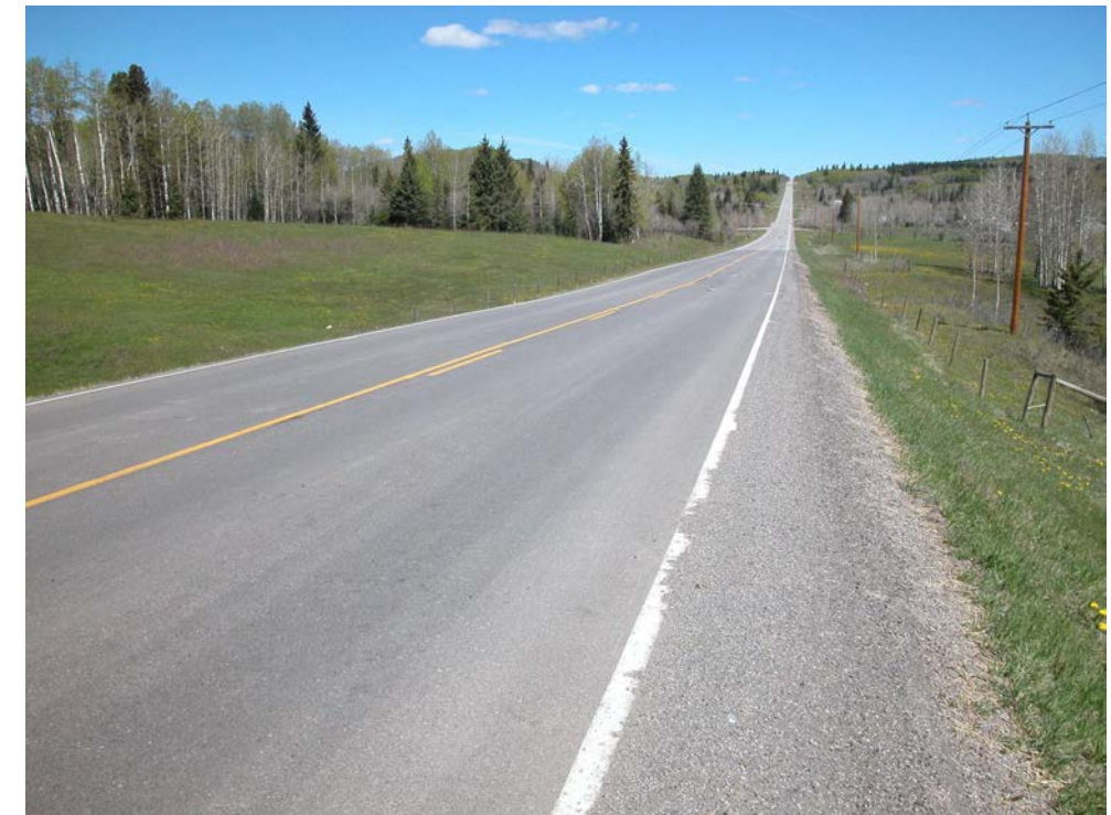
Photo S10C-2 (upper right) – May 2004 – Another view of the July 2003 overlay at Site C, facing north. No recent cracking noted in the road surface.
