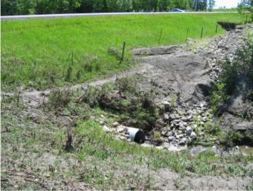
Photo S10(C)-5 (above) – June 2005 – erosion damage in west ditch, south of the culvert.
