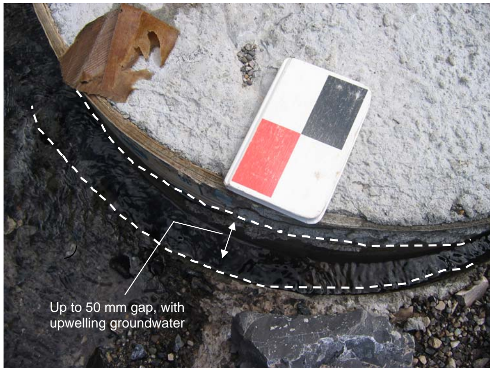
Photo S15-3 (lower left) – May 2006 – open gap along the east side of the east anchor pile for the barrier. It appeared that the pile had been pulled towards the west with up to approximately 50 mm lateral displacement at ground surface. It also appeared that there was groundwater discharge upwelling around the pile at the time of the inspection.
