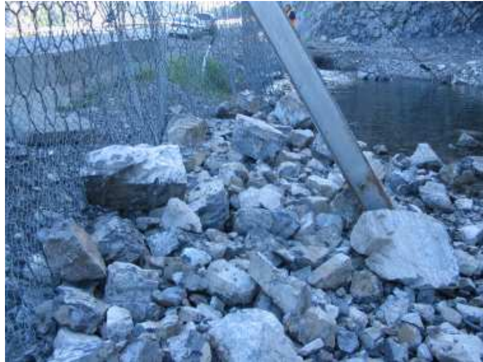
Photo S15-4 – June 2007 (upper left) Rockfall debris that has accumulated around the base of one of the barrier support posts. This post also appeared to be leaning too far forwards, compared to design angle of 15° from vertical.
