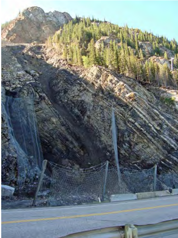
Photo S15-3 (top left) – June 2009 The gully erosion in the talus slope above the net has expanded since the 2008 inspection (the left gully fork). Compare with Photo S15-5.
