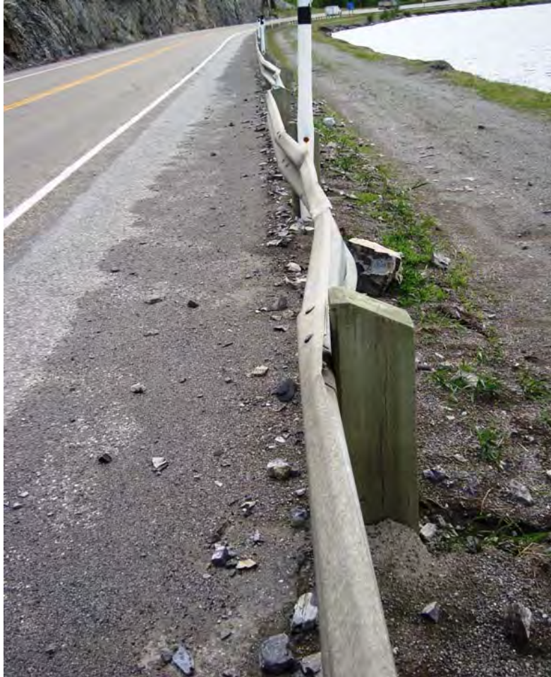
Photo S15-2 (June 2012) – Facing towards the southwest at the guardrail where impact damage has occurred. Numerous rock fall debris ranging from gravel to cobble size was present along the road shoulder.
