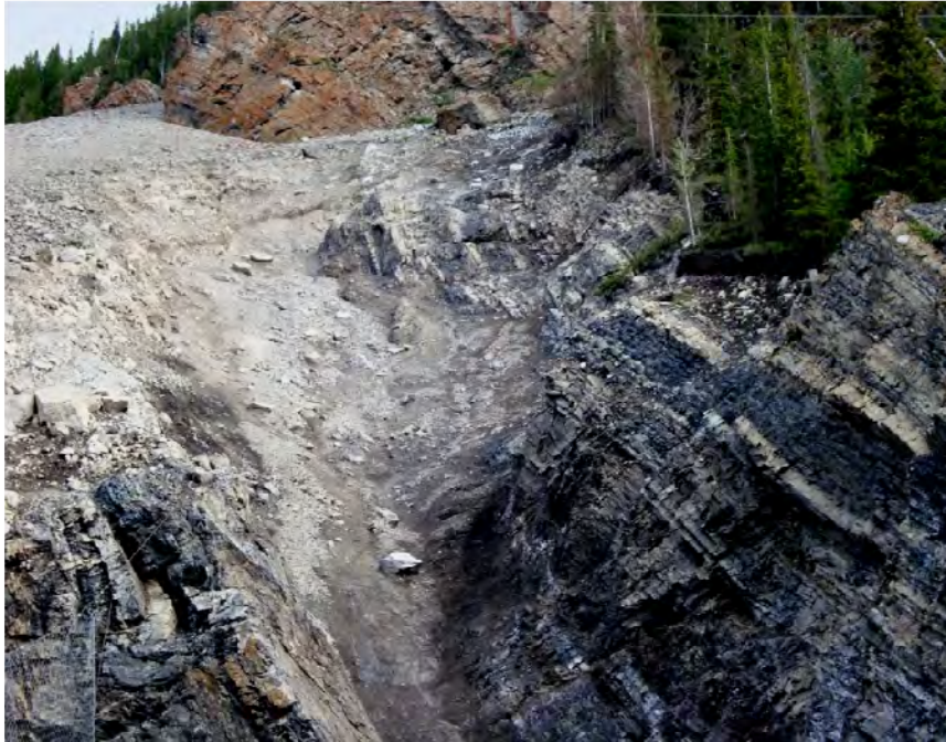
Photo S15-3 (June 2011) – The upper gully in the talus slope as observed during the 2011 inspection.
