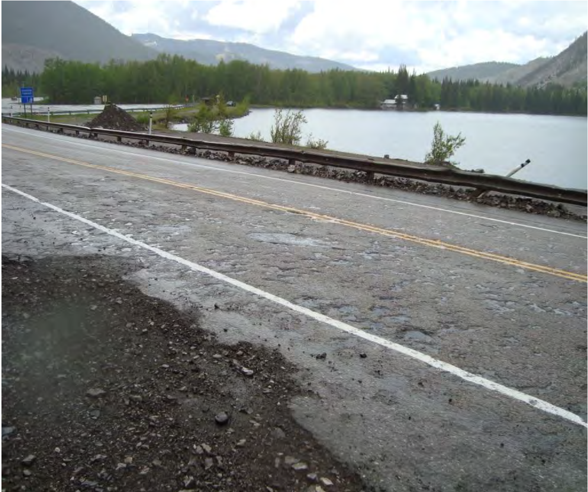
Photo S15-5 (May 2013) – Impact damage of the road surface and guardrail west of the barrier net due to falling rock from recent scaling work.
