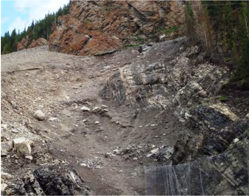
Photo S15-6 (June 2012) – The upper gully in the talus slope as observed during the 2012 inspection.
