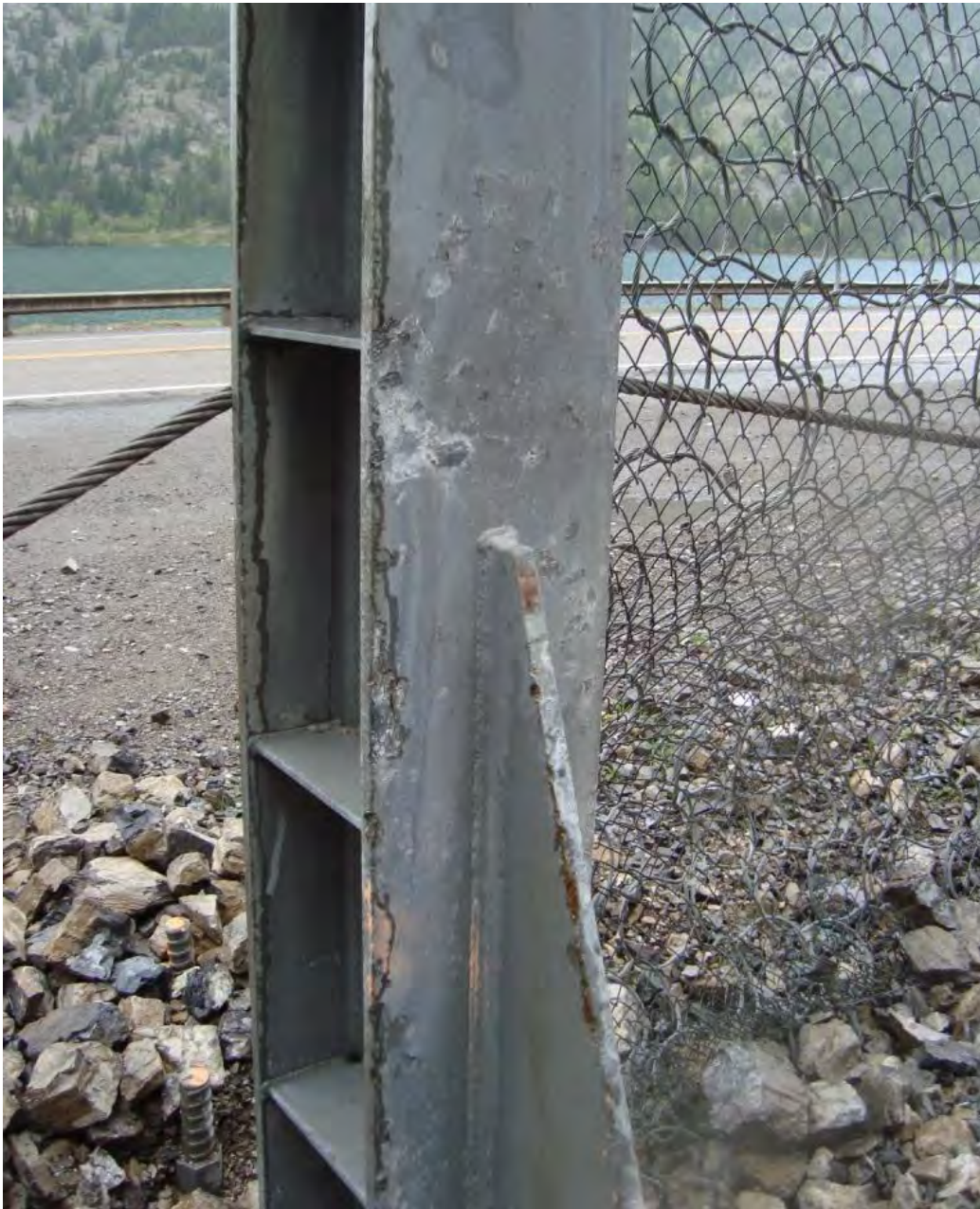
Photo S15-2 (May 2013) – The support post of the barrier net showing minor damage from rock fall impacts
