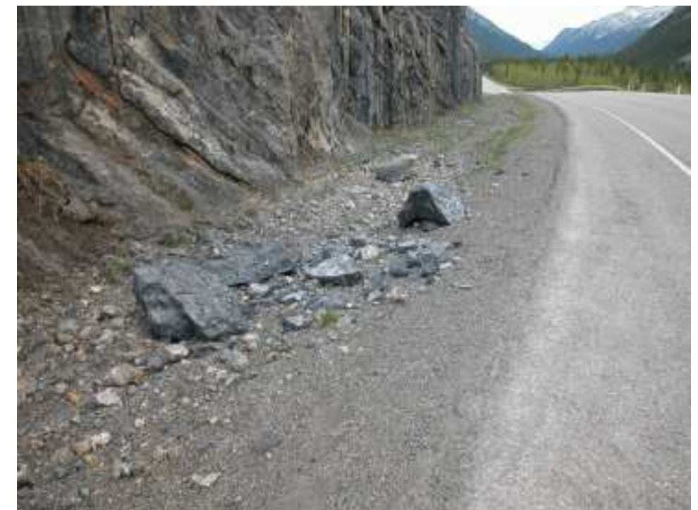
Photo S18-7 – June 2004 (lower right) Boulder-sized rockfall debris in the ditch near the central portion of the East Cut Slope as seen during the June 2004 site inspection. The ditch in this area is typically 4 m or less in width and 0.5 to 0.75 m in depth, which does not meet the recommended ditch sizing criteria.
