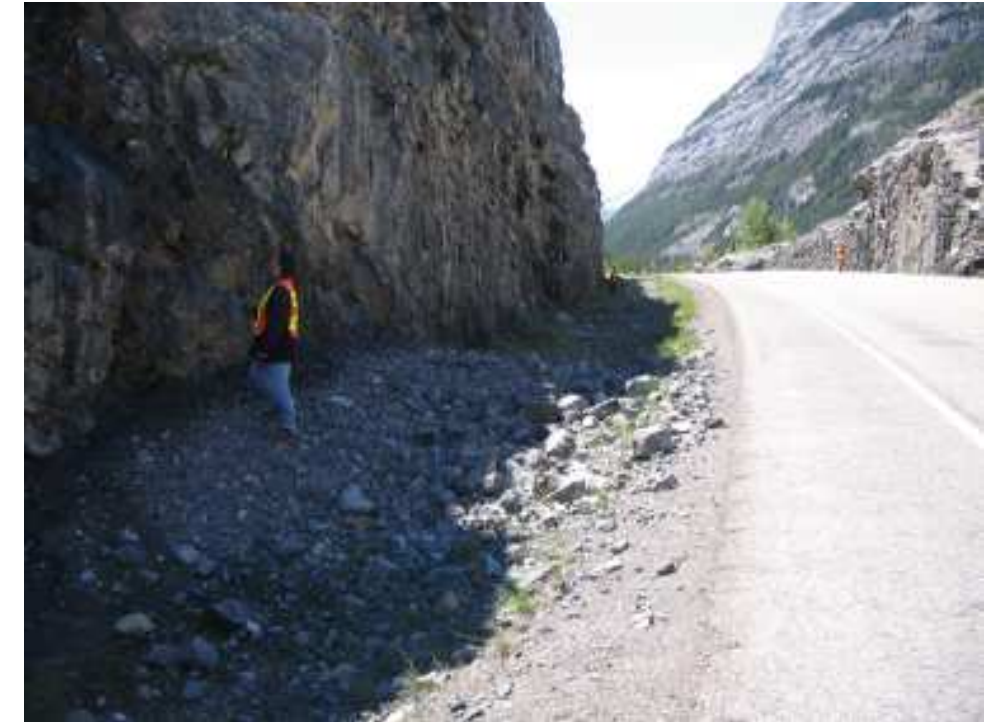
Photo S18-5 – June 2007 (upper right) Facing southbound along the east edge of Highway 40 in the central/northern portion of the East Cut Slope. Note the relatively greater accumulation of rockfall debris in this area compared to the segment of the ditch further south (Photo S18-4). Some of the rocks have been deposited along the edge of the pavement. A few gravel-sized pieces of rock were noted on the pavement at the time of the inspection, and cobble-sized rocks were noted near the centerline of the road in the June 2004 inspection.
