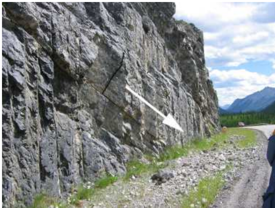
Photo S18-6 – 2005 (lower left) This photo from a 2005 site recon during the highway corridor geohazard review illustrates one of several locations along the East Cut Slope where large rockfalls are developing due to weathering and freeze/thaw effects in open cracks. At this location, the large boulder in front of this open crack will break free in the future and fall outwards into the ditch. If this large piece of rock falls out as one piece, the resulting debris could encroach onto the road and/or cause subsequent debris to bounce and roll onto the road.
