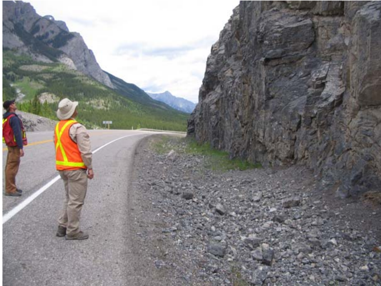
Photo S18-3 (top) – June 2008 Facing northbound along the east highway ditch in the north end of the site. There was a considerable accumulation of rockfall debris from the East Cut Slope in the ditch in this area, with gravel to cobble sized particles onto the edge of the pavement.
