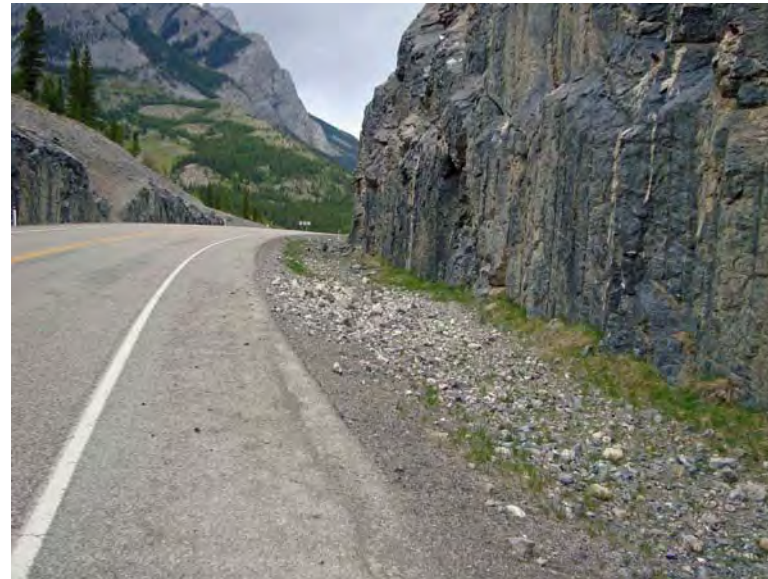
Photo S18-5 – June 2009 Facing northbound along the east ditch near the centre of the rock cut. Area of greatest rockfall where rock has likely landed on the road.
