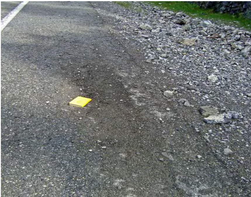
Photo S18-5 – June 2012 Standing at approximately the center of the site on the west side of the road looking northbound. There is apparent damage to the west road shoulder from current rock falls and/or a gravel slide that occurred during the 2011/2012 winter season.
