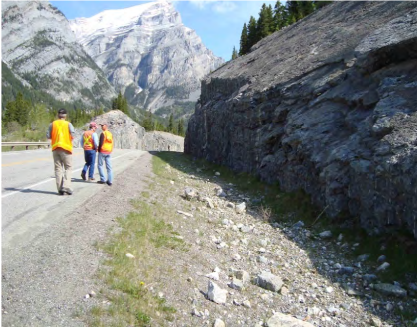
Photo S18-2 – June 2010 Facing northbound along the east ditch near the south end of the East Cut. Minor rock fall in this area that does not appear to have landed on the road; however boulder and cobble-sized rocks have been noted onto the edge of the pavement in past inspections.
