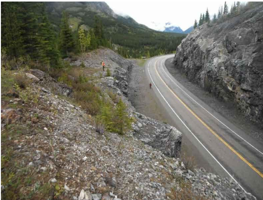
Photo S18-3 – May 2013 Facing northbound from the top of the West Cut Slope. All rock fall was contained within the ditch.
