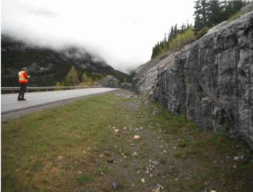
Photo S18-2 – May 2013 Facing northbound along the east ditch near the south end of the East Cut. Minor rock fall was observed in this area that did not appear to have landed on the road.
