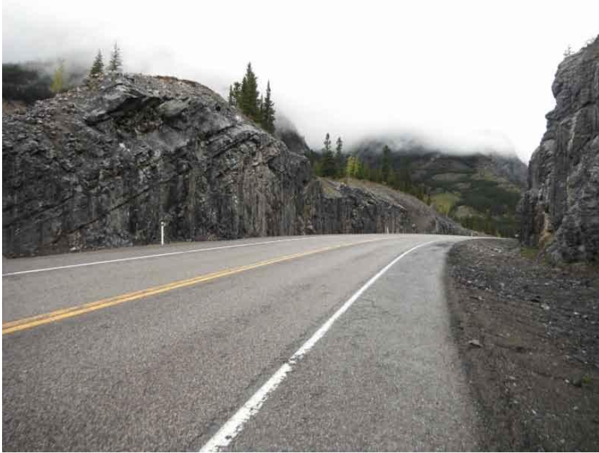
Photo S18-4 – May 2013 Standing at approximately the center of the site on the east side of the road facing northbound. Rock fall impacts were observed on the east road shoulder.
