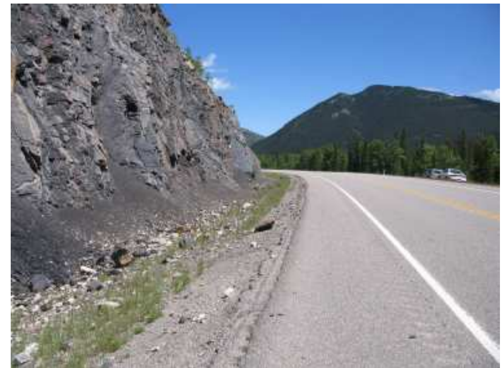
Photo S20-6 – June 2007 (lower right) Facing eastbound across the north ditch at the east end of the cut slope. Relatively less rockfall debris was present in the ditch at this end of the site, however some cobble-sized rocks were still noted within 1 m of the edge of the pavement.
