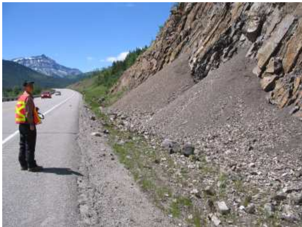
Photo S20-5 – June 2007 (lower left) Facing westbound across the area shown in Photo S20-4.
