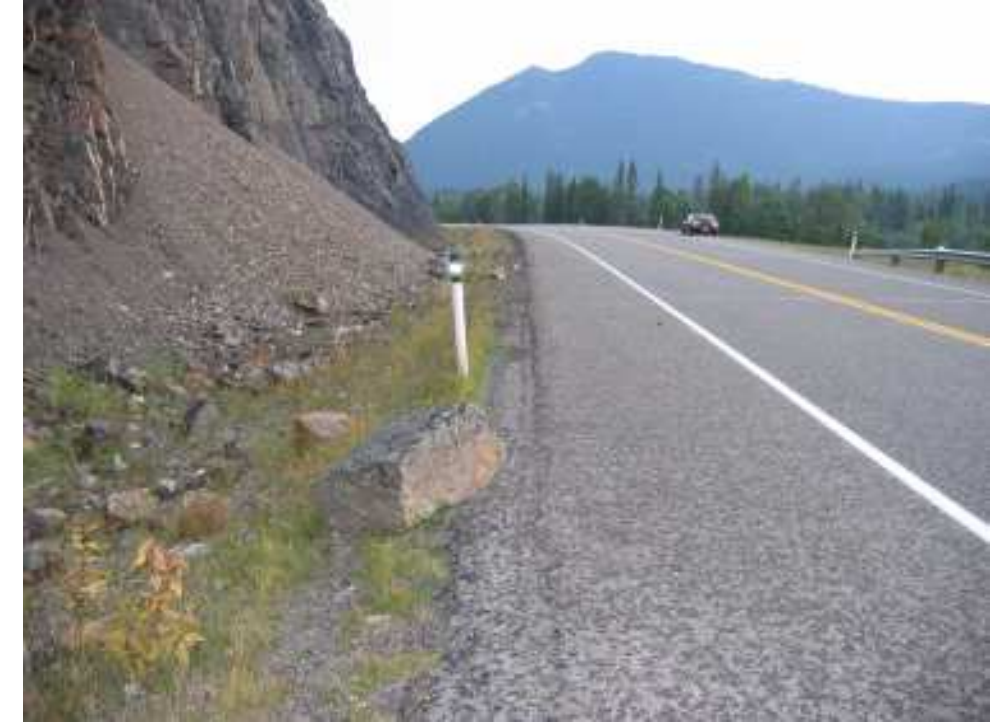
Photo S20-8 – August 2004 (upper right) Boulder sized rockfall debris deposited along the north edge of the pavement in the central/west portion of the site.
