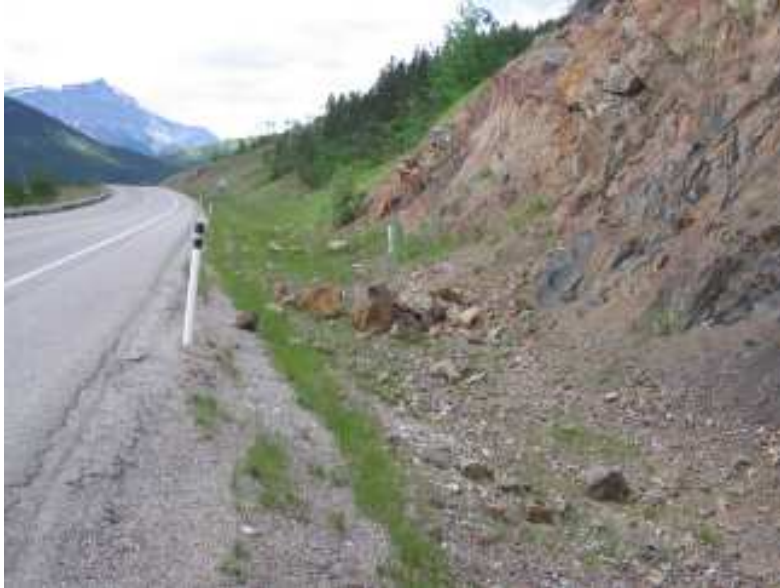
Photo S20-1 (top) – June 2008 Facing westbound across the far west end of the site. Note the boulder sized debris that has fallen into the ditch.
