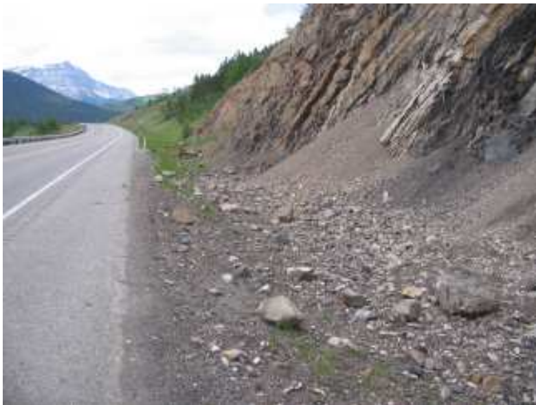
Photo S20-2 (bottom) – June 2008 Another view facing westbound from the west end of the site and from below the gully/chute in the slope above the crest of the cut. Note the accumulation of rockfall debris in the ditch, including cobble sized rocks near the edge of the pavement. Several gravel sized rocks were found on the pavement during the 2008 inspection, and during previous inspections up to cobble sized rocks were noted on the pavement.
