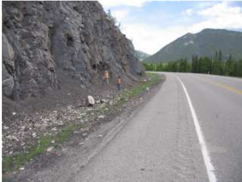
Photo S20-3 (top) – June 2008 Facing eastbound from the central portion of the site, showing the accumulation of rockfall debris in the ditch east of the area below the chute.
