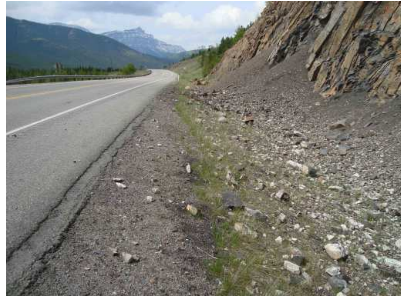
Photograph S20-3 – Looking westbound along the north ditch. Note the large boulders that have rolled down the main debris cones to within 2 m of the paved surface at the time of the June 2010 inspection.
