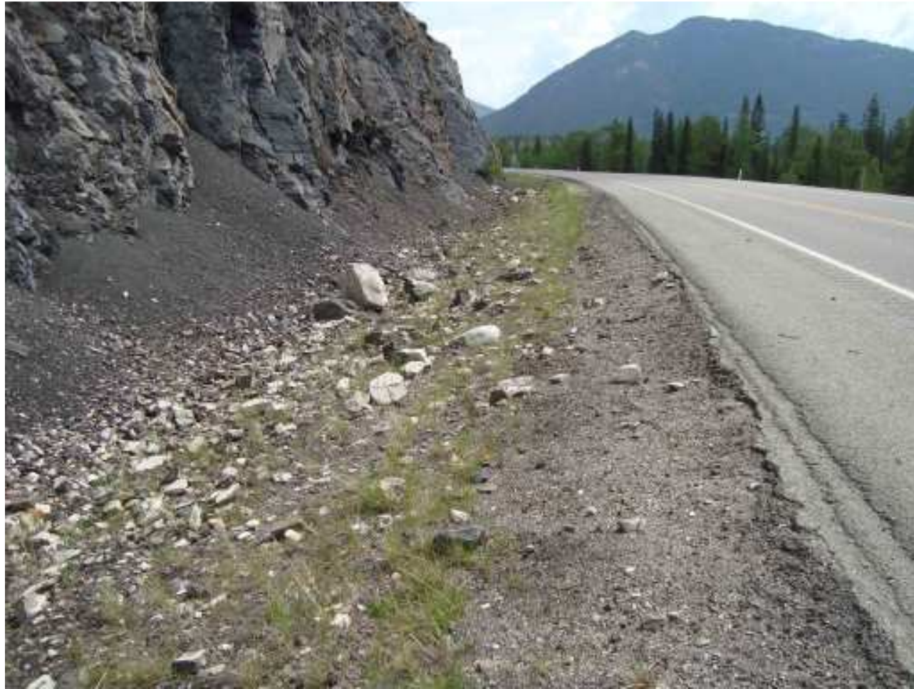
Photograph S20-2 – Looking eastbound along the north ditch. Rock fall includes gravel to cobble sized rocks, with gravel on the paved shoulder and cobbles immediately adjacent to the paved surface. Boulder sized rocks are also present in the ditch, and during past inspections have been noted at positions along the edge of the pavement.
