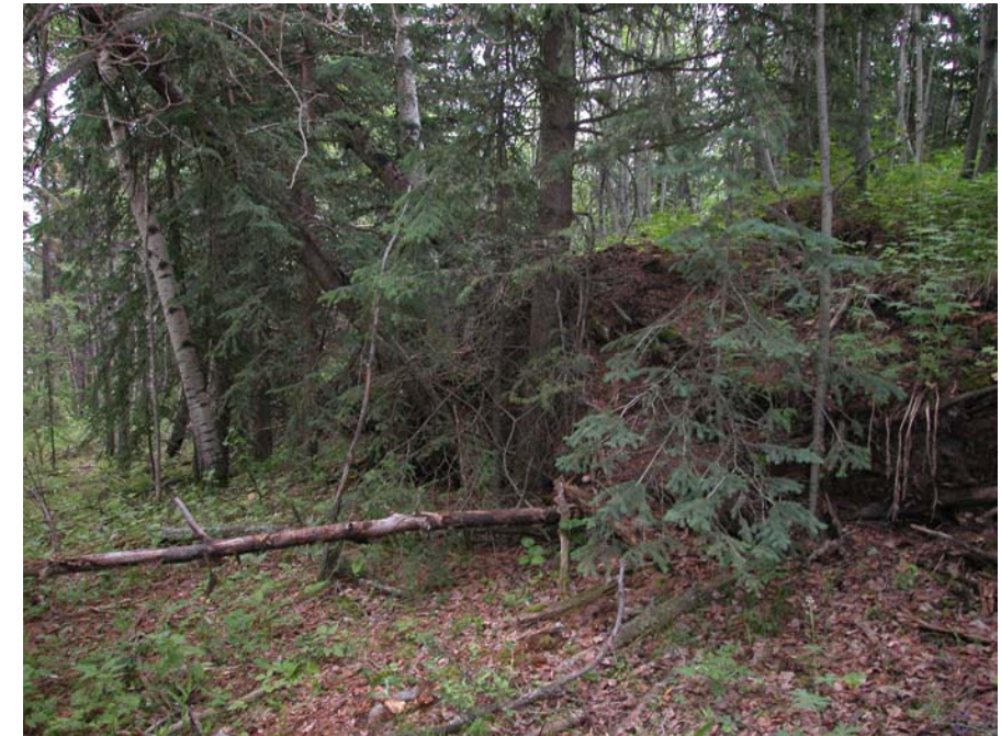
Photo 4 (upper left) – July 2003 Facing east along the north shoulder of the road through the slide area. Note the loss of ground immediately downslope of the guardrail. The existing pile wall along the north shoulder of the road remains partially effective in supporting the shoulder, however ongoing movement of the slide below the road has still resulted in continued settlement and cracking of the road surface and deformation of the guardrail, as shown in Photos 1, 2 and 3.
