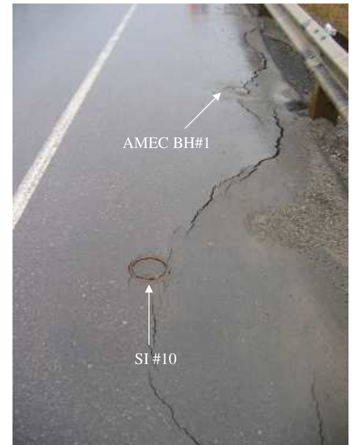
Photo S2-4 (lower right) – June 2005 – Cracking in the westbound lane passes right next to SI#10 and AMEC BH#1. The instruments were read in May 2005 and prior to the development of the cracks.
