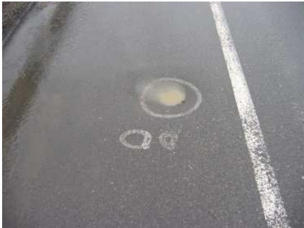
Photo S2-7 (lower left) – June 2005 – SI#9 on road surface. Repeated repavings have left SI's #9, #10, and #11 below the road grade and difficult to access. The protective cover over the SI in AMEC BH#1 was also damaged by repaving in 2004 and can no longer be removed to read the SI.
