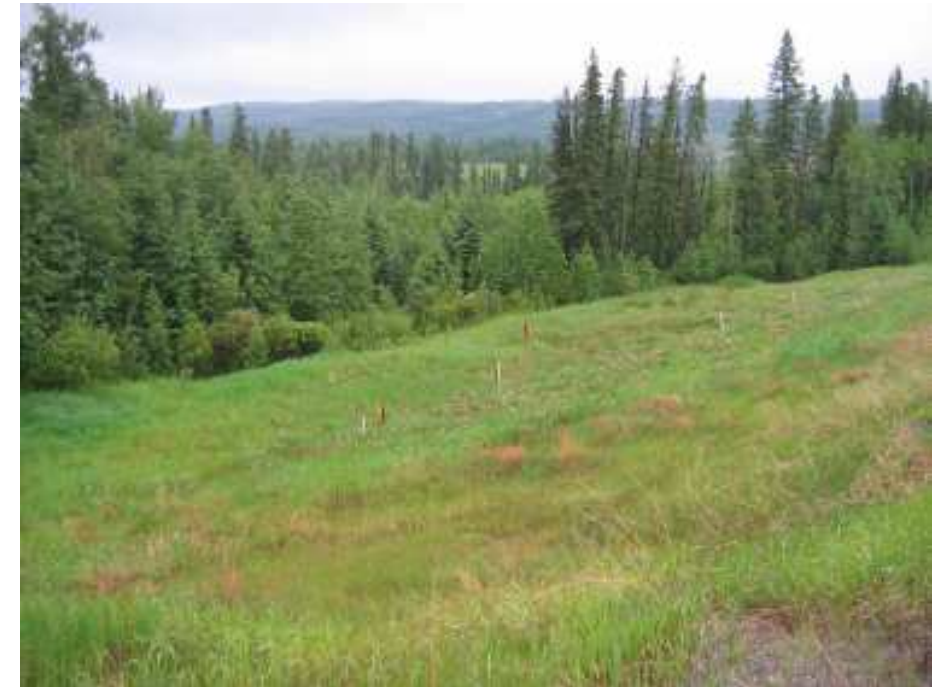
Photo S2-6 (upper right) – June 2005 – General view of the slope face below the road with instruments visible near the toe of the slope.
