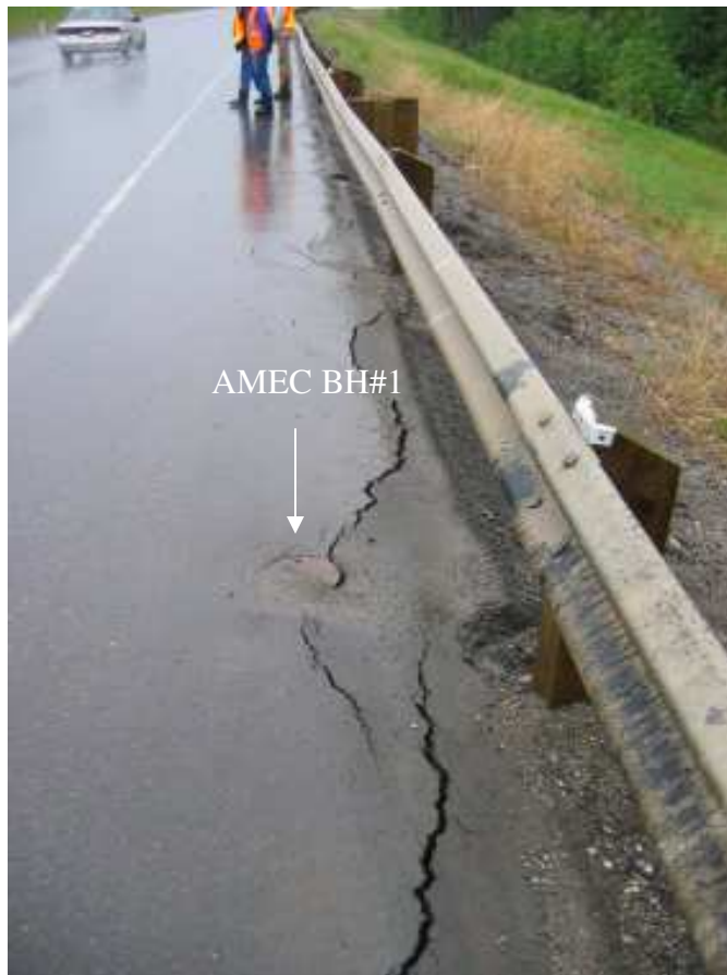
Photo S2-3 (lower left) – June 2005 – Closer view of cracking in the westbound lane. Note the downslope movement of the guardrail post evidenced by the edge of the asphalt.
