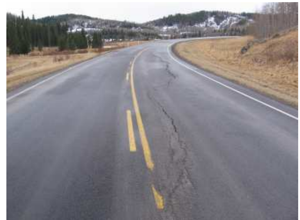
Photo S22-3 – March 2007 (lower left) Another view of the cracked area shown in Photos S22-1 and 2, as seen in March 2007 during the borehole drilling and instrument installations. This photo was taken prior to the June 2007 overlay and illustrates the degree of cracking and settlement that had developed in this area. A similar degree of damage had formed at this location in recent years but has been treated as a maintenance concern with repeated overlays and patching.
