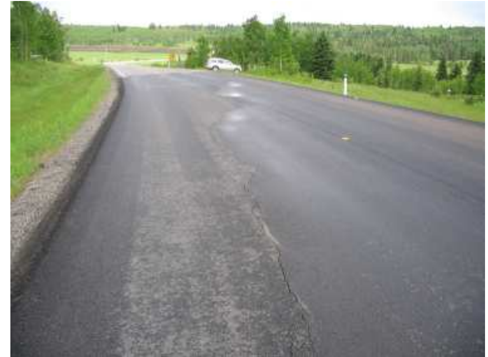
Photo S22-1 – June 2007 (upper left) Facing southwest along the highway near boreholes 2007-7 and 2007-8, which are on the shoulder of the road just beyond the delineator post visible on the left. An overlay was placed across the entire road width a short time before the site inspection and the visible crack across the southbound lane and part of the northbound lane has formed since the overlay. Significant cracking and settlement was noted at this same location before the recent overlay – see Photos S22-3, 4 and 5.
