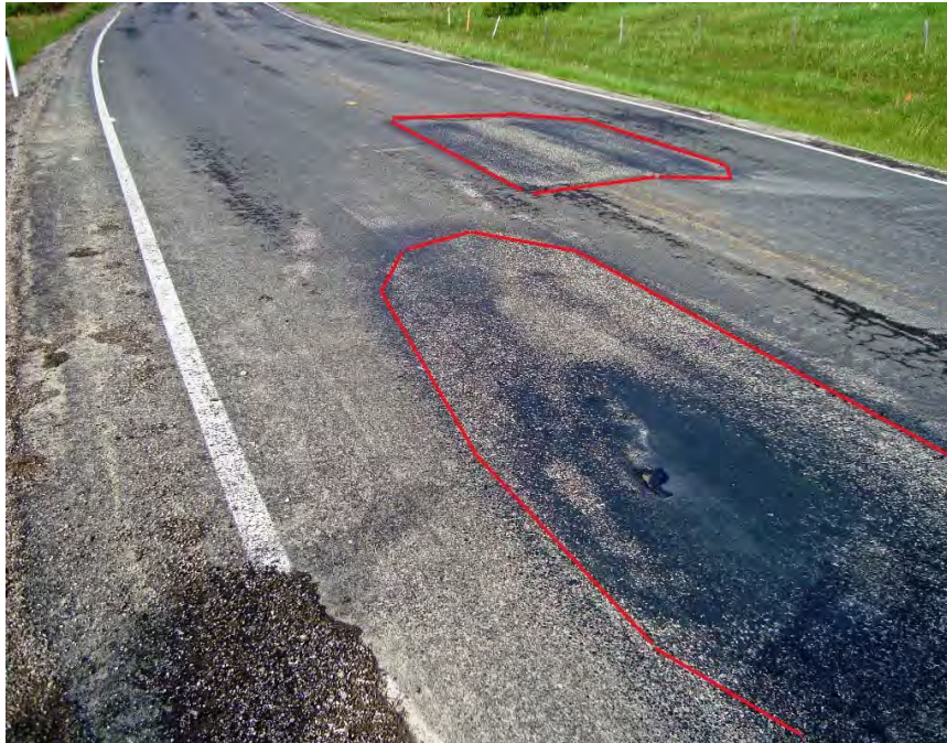
Photo S22-1 – June 2012 Facing west (along the southbound lane) from the east end of the site. The recent milling work has exposed asphalt experiencing sub-grade failure (outlined in red). Milling may have caused the sub-grade failure.
