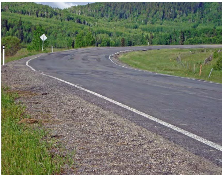
Photo S22-2 – June 2012 Facing west (along the southbound lane) from the east side of the site. The damage to the road surface is similar to that noted during past inspections.
