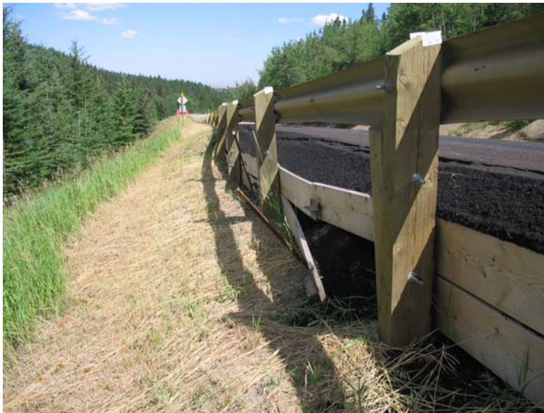
Photo S26-6 (bottom) Timber lagging installed along the upslope edge of the guardrail at the north flank of the damaged segment of the highway. The accumulated thickness and weight of the multiple overlays has caused the lagging to bulge outwards.
