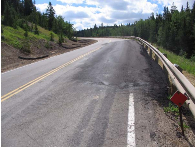
Photo S26-5 (top) Another view of the damaged segment of the highway, facing southbound.
