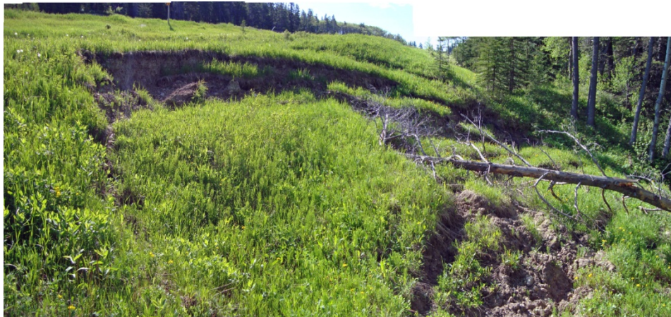
Photo S26-7 – bottom - (June 2011) A slump on the lower slope at Area A extending to creek level. The slump was active during 2010.
