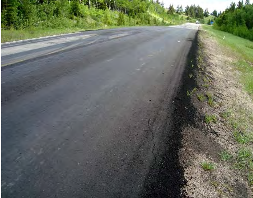
Photo S26-1 - (June 2012) Facing south from the south end of Area A at the west road shoulder. Overlays have been placed at the damaged areas recently. Minor cracking was visible along the shoulder through the new overlay.
