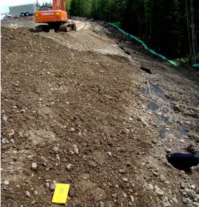
Photo S26-4 - (June 2012) Facing southwest from the lower west slope at Area B. Construction was underway during the inspection.
