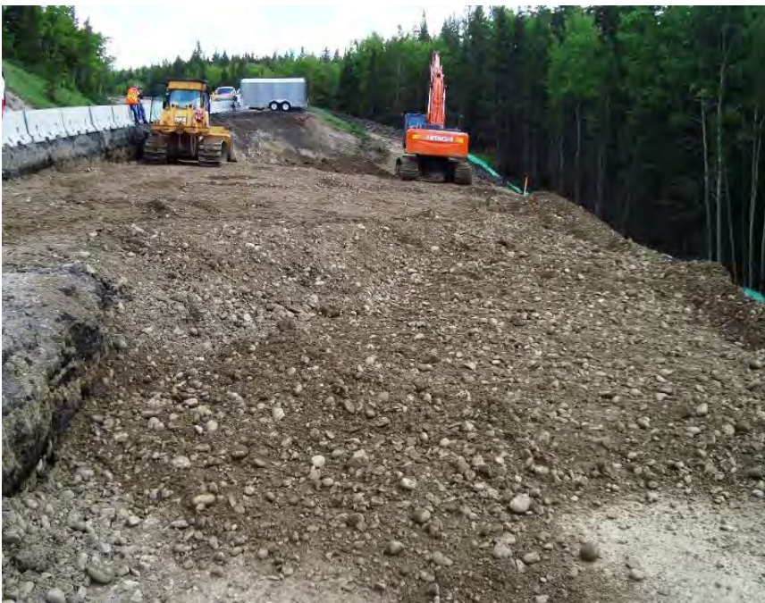
Photo S26-5 - (June 2012) Facing south from the upper slope on the west side of Area B. Construction of the shear pile repair was underway during the inspection.
