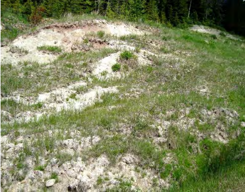
Photo S26-3 - (June 2012) Facing southeast from the north end of Area A at the seepage area on the east side of the highway. The ditch here was blocked with soil as a result of ongoing back slope movement.
