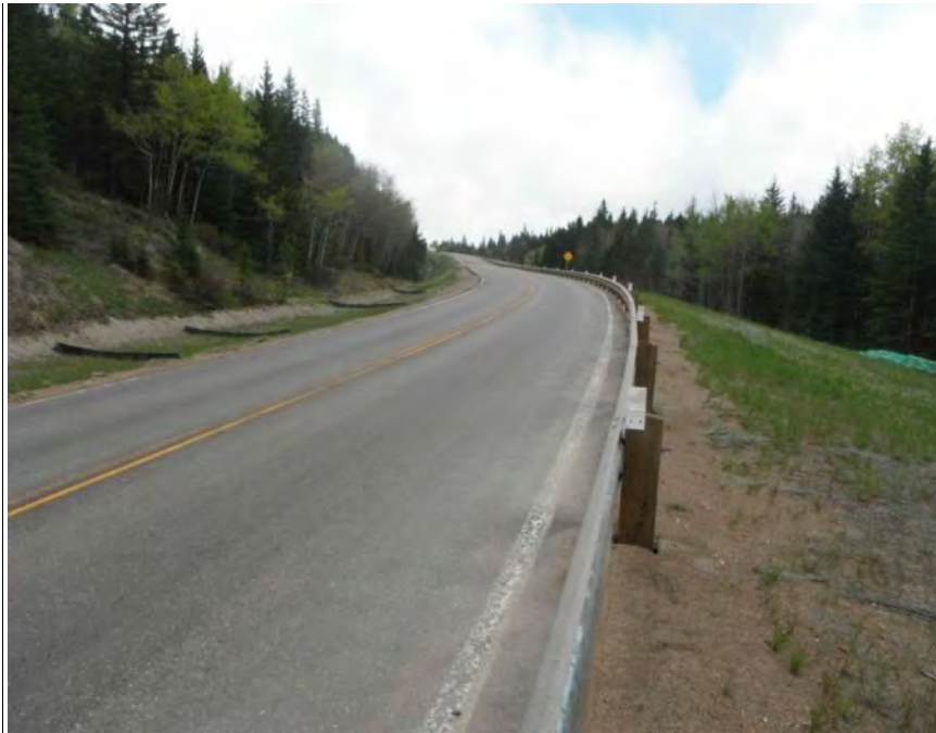
Photo S26-3 - (May 2013) Facing south from the west side of Area B. No new cracking or settlement was observed on the road surface.
