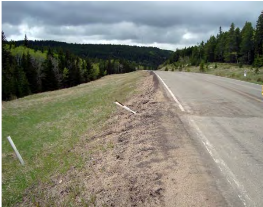
Photo S26-1 - (May 2013) Standing near the culvert outlet at Area A at the southern edge of the site looking towards the northwest. Numerous overlays and patches have created a drop-off on the downslope road shoulder northwest of the culvert.
