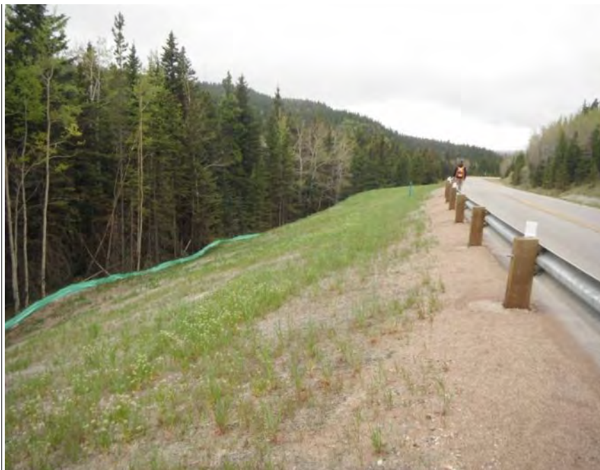
Photo S26-4 - (May 2013) Facing south from the upper slope on the west side of Area B. Construction of the shear pile repair was complete in Fall 2012. Vegetation has begin to grow during 2013 inspections.
