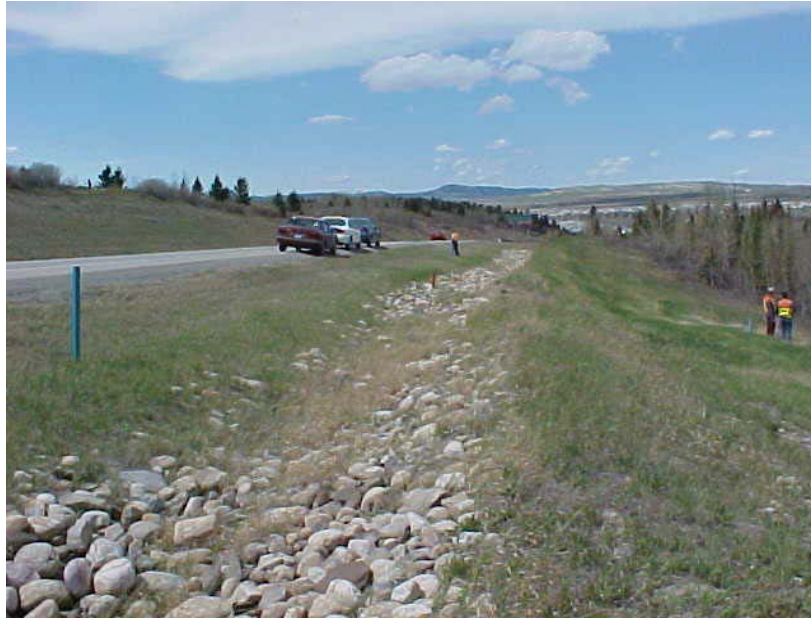
Photo 1 – May 2002 photo of ditch along downslope edge of highway showing area where ditch liner was repaired in summer 2000. Repairs continue to function adequately.
