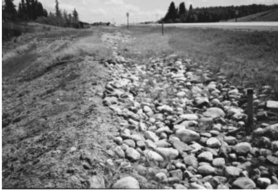
Photo 1 – Ditch along downslope edge of highway showing area where ditch liner was repaired in summer 2000. Effective drainage should be maintained to minimize the amount of surface drainage entering the slide area.
