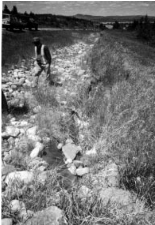
Photo 2 – June 2000 photo showing damaged ditch liner. The damage to the liner likely allowed surface drainage to flow into slide area, possibly exacerbating movements.
