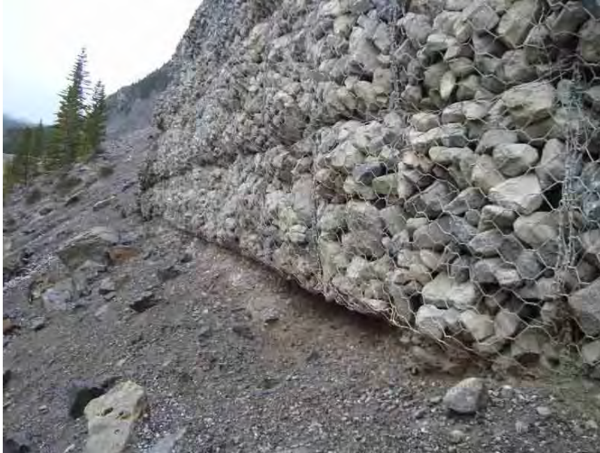
Photo S30-3 – May 2013 Undermining at the base of the northeast end of the gabion wall. There was no flow at the time of the site inspection but the soil was wet.
