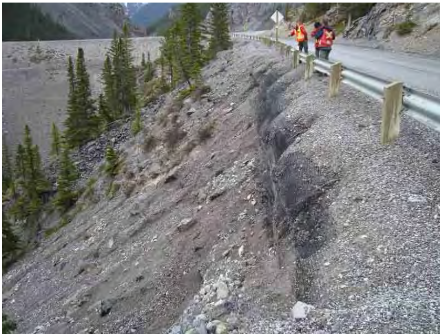
Photo S30-4 – May 2013 Erosion along the downslope edge of the highway, above the collapsed segment of the wall. The geogrid within the road embankment continues to support the highway, but the loss of erosion protection provided by the gabion wall has allowed surface erosion to continue. Since the previous inspection, the erosion has retrogressed onto the shoulder and approximately 200 mm past the guard rails.
