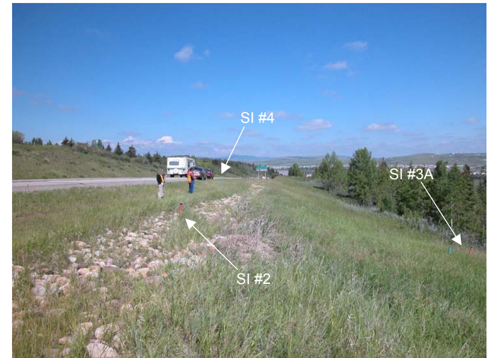
Photo 8 (right) – July 2003 Facing west along ditchline parallel to north shoulder of Highway 22. Repairs to the ditch liner continue to function adequately, however it appears that some relatively low gradient/high spots in the ditch may be allowing water to pool in the ditch and possibly overflow during peak flow times – leading to the development of the minor gully (shown in Photo 5) leading into the shallow sliding area at the fenceline.
