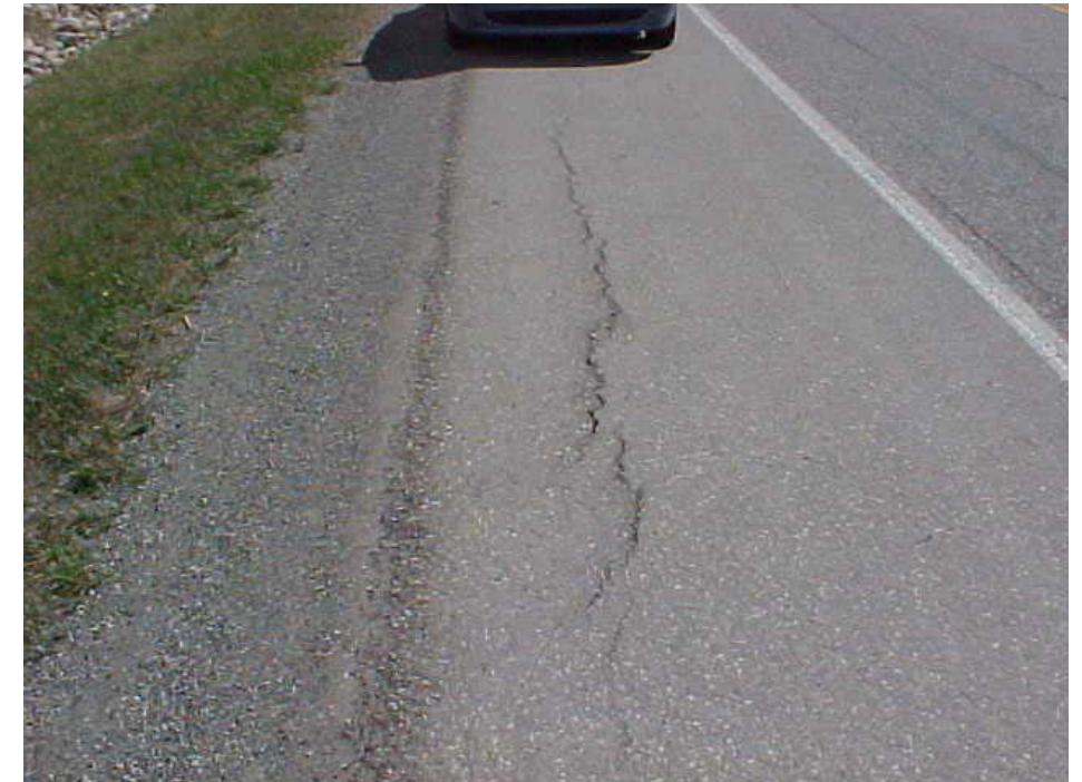
Photo 2 (upper right) – May 2002 Same area as shown on Photo 1, as seen during May 2002 inspection.
