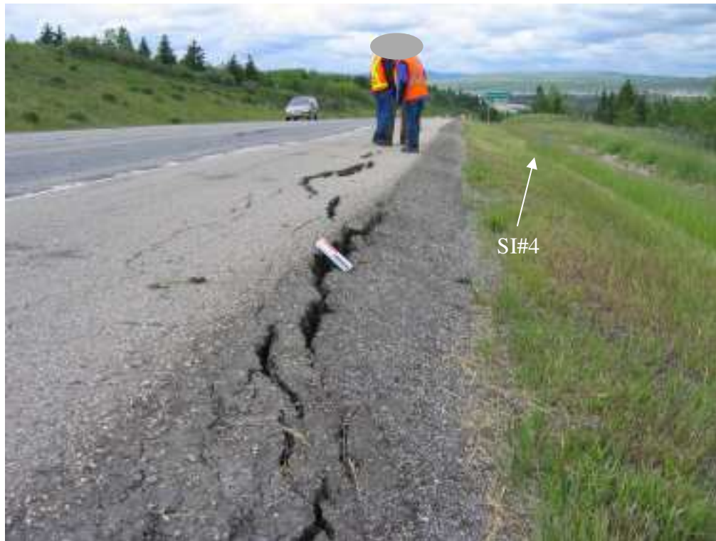
Photo S3-4 (upper left) – June 2005 – facing west along the road. Large cracks in the shoulder developed between the time of instrument readings in May 2005 and the site inspection in late June 2005.
