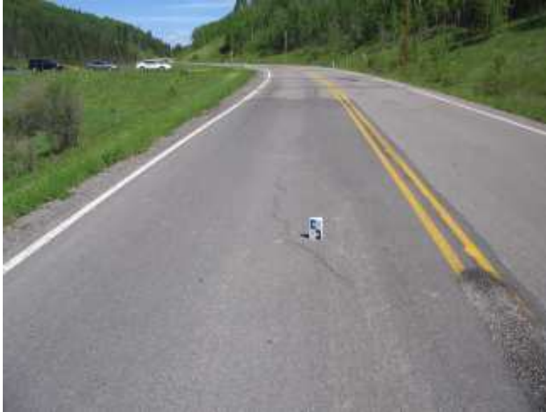
Photo S31-3 (top) – June 2008 Facing north in the north end of the overlays, with recent cracking and very minor settlement of the road surface visible in the southbound lane. The position and pattern of these cracks suggest that they are the north flank of overall circular cracking roughly centered around the culvert outlet visible on the slope face below the road.
