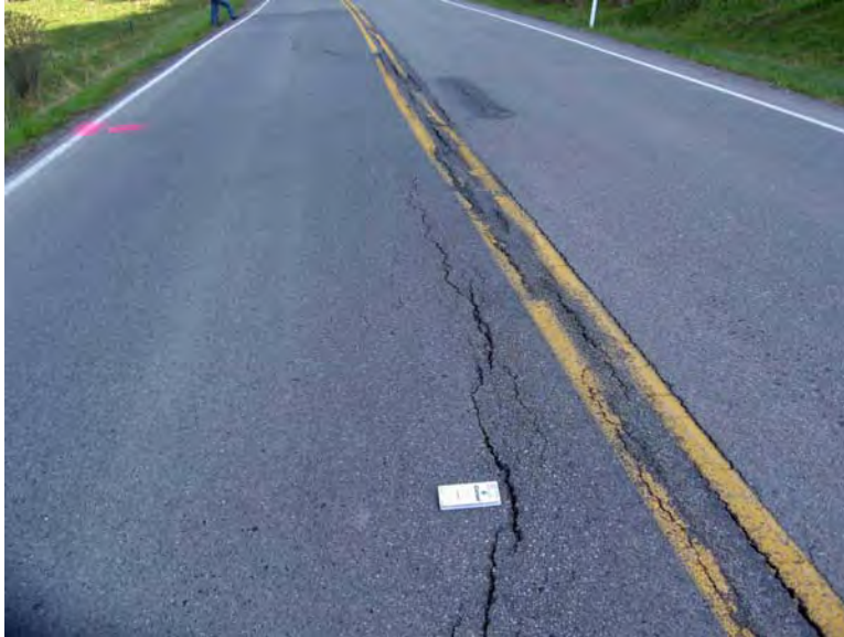
Photo S31-3 – June 2009 Close-up view of the cracking taken from the south facing north. Planned SI location marked on pavement (pink paint marking).
