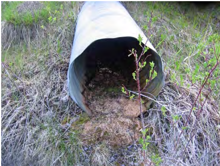
Photo S31-4 – June 2009 The culvert outlet was not flowing at the time of the inspection but appeared to have carried water recently.
