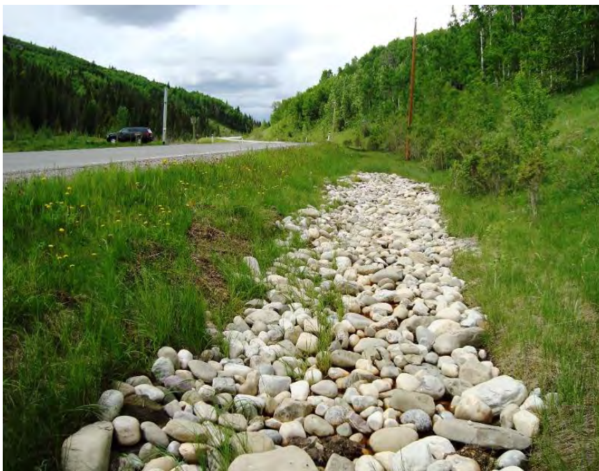
Photo S31-2 (June 2012) Facing north from the center of the site in the east upslope ditch. Cobbles were placed in the ditch in an approximately 80 m long segment. The new drainage pipe inlet was buried beneath the cobbles.
