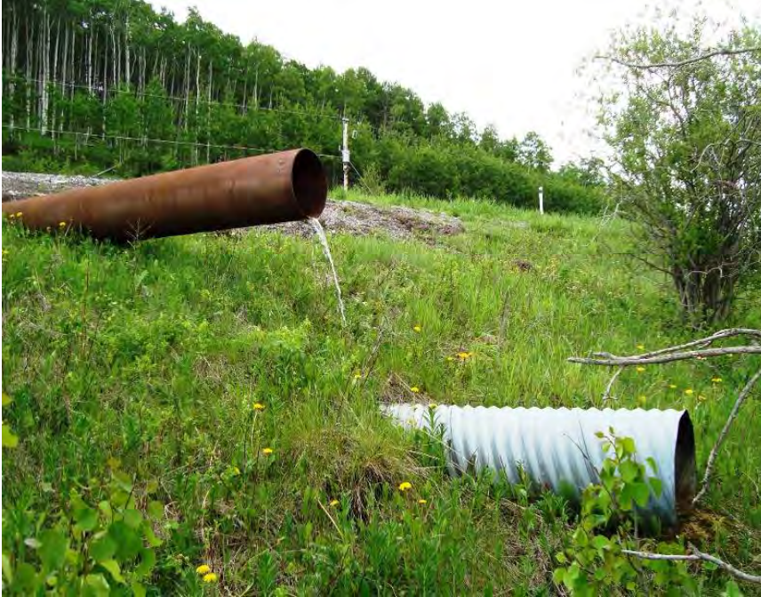
Photo S31-3 (June 2012) Facing southeast from the bottom of the west embankment. The new drainage pipe is visible and flowing at approximately 10 L/min (brown pipe). The previous culvert is visible below it and was not flowing. The overhang of the new drainage pipe forms an obstruction hazard in the west ditch.
