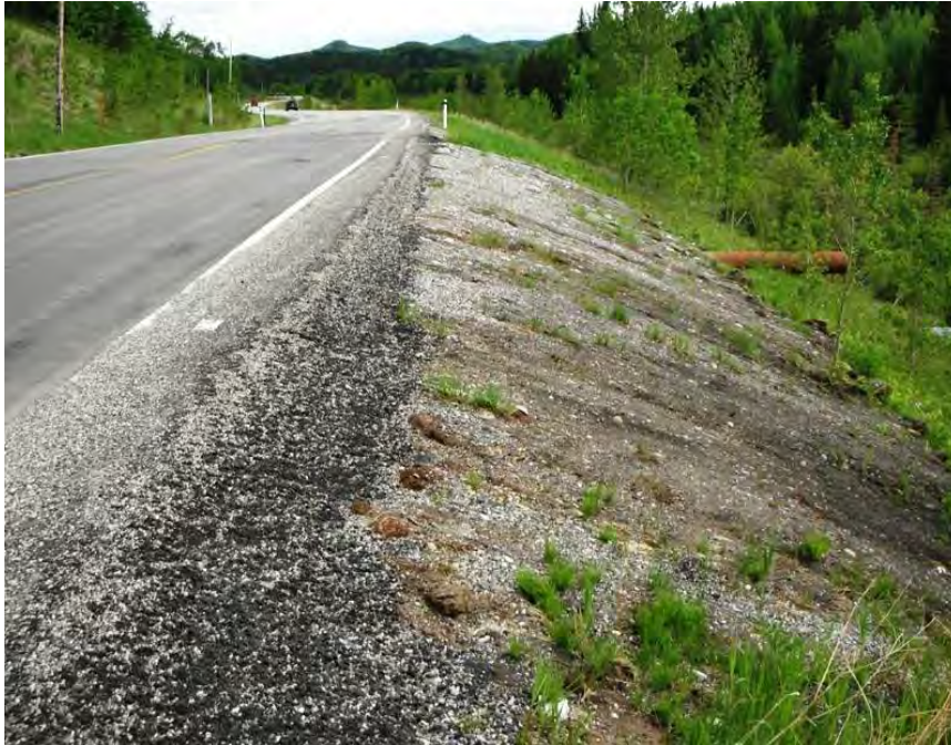
Photo S31-1 (June 2012) Facing south from the north end of the site. This segment of the road was apparently excavated and rebuilt. A new drainage pipe was installed underneath the road. The outlet is visible on the right hand side of the photo (brown pipe). Subtle settlement was visible along this segment of the highway in previously noted areas of cracking.
