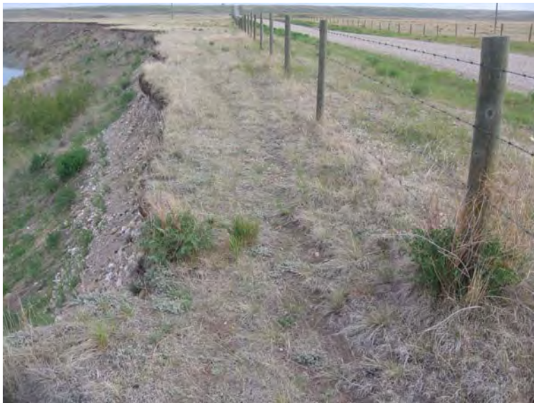
Photo S32-2 (bottom) – June 2009 Closer view of the area of minimum offset between the slope crest in the landsliding area and the highway. The minimum offset was measured to be 1.6 to 1.7 m in June 2009, compared with 1.7 m in June 2008.
