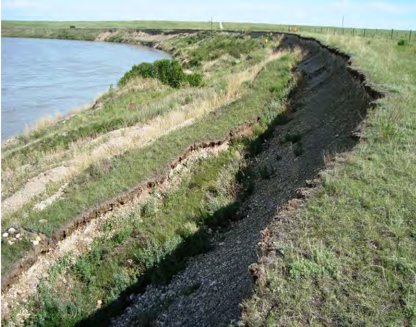
Photo S32-3 – June 2012 Facing north over the main landslide area. Some evidence of fresh sliding was observed but the main crest is mainly unchanged from the 2010 inspection.
