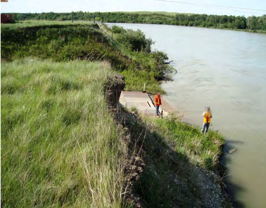
Photo S32-1 – June 2012 Facing south towards the east ferry ramp. The ferry guide wire support tower is just out of the frame on the left side of the photo. This area appears mostly unchanged since the previous inspection.
