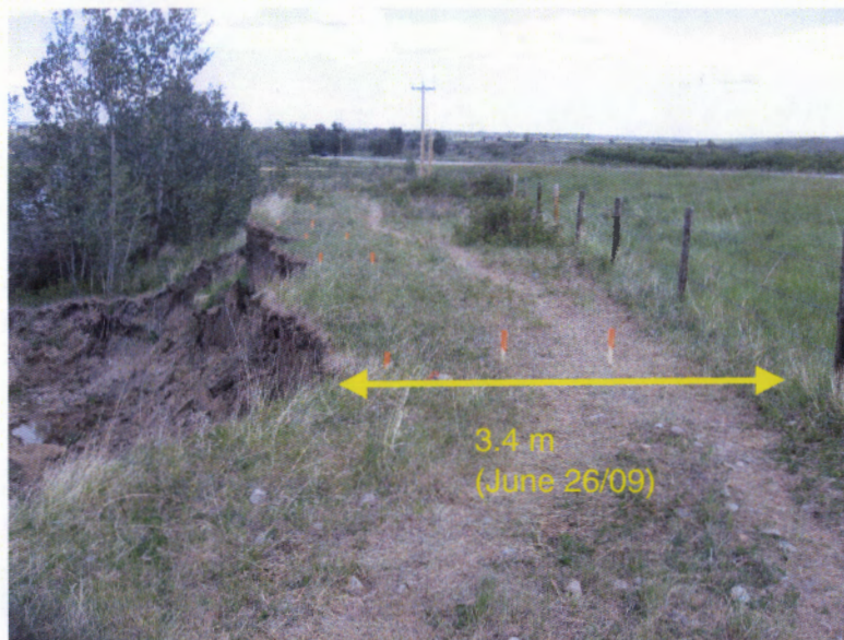
Photo 4 (bottom) – View north along the slope crest, at the point of maximum retrogression towards the highway (offset 3.4 m from the fenceline). Reference stakes were placed at selected locations along the slope crest, at 0 and 1 m offset along with a third stake at 2 m offset at the location shown.
