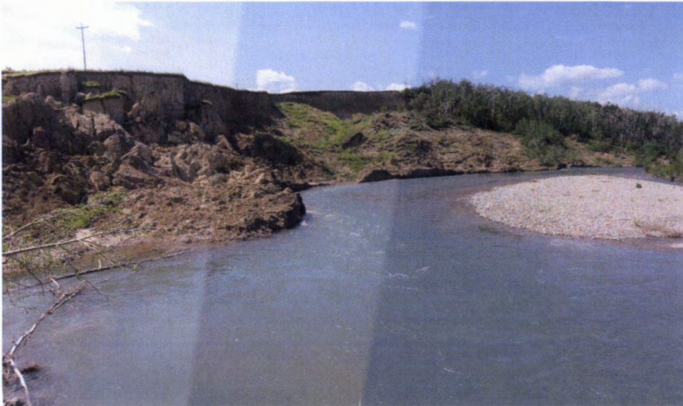
Photo 3 (top) – View upstream towards the toe of the landslide area. Photo is taken from the downstream end of the meander loop and on top of the armored right bank downstream of the landslide area that is being outflanked and eroded. Note the significant toe bulge/thrust from the recent landsliding.
