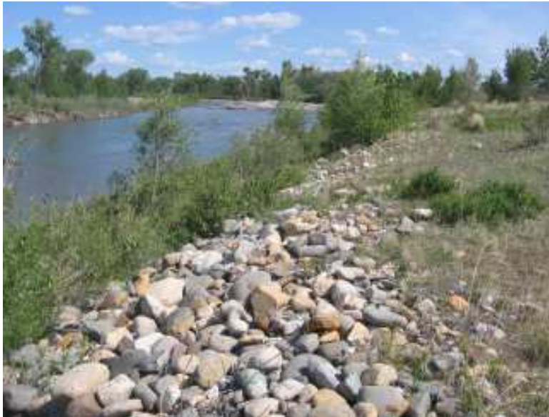
Photo 5 (top) – View downstream of the armored right bank, which is located downstream of the meander bend and landslide area. The upstream end of this armored segment of the bank is being outflanked and eroded by the meander bend.
