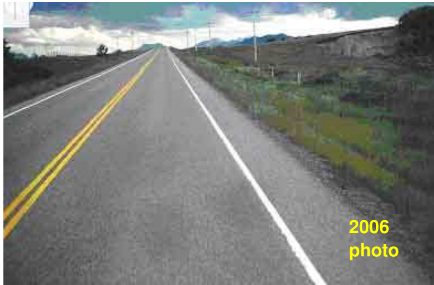
Photo 7 (top) – Photo from 2006 videolog provided by AT, facing southbound along the highway adjacent to the landslide area. Note the significantly greater offset between the crest of the slope and the highway compared to the June 2009 photos.
