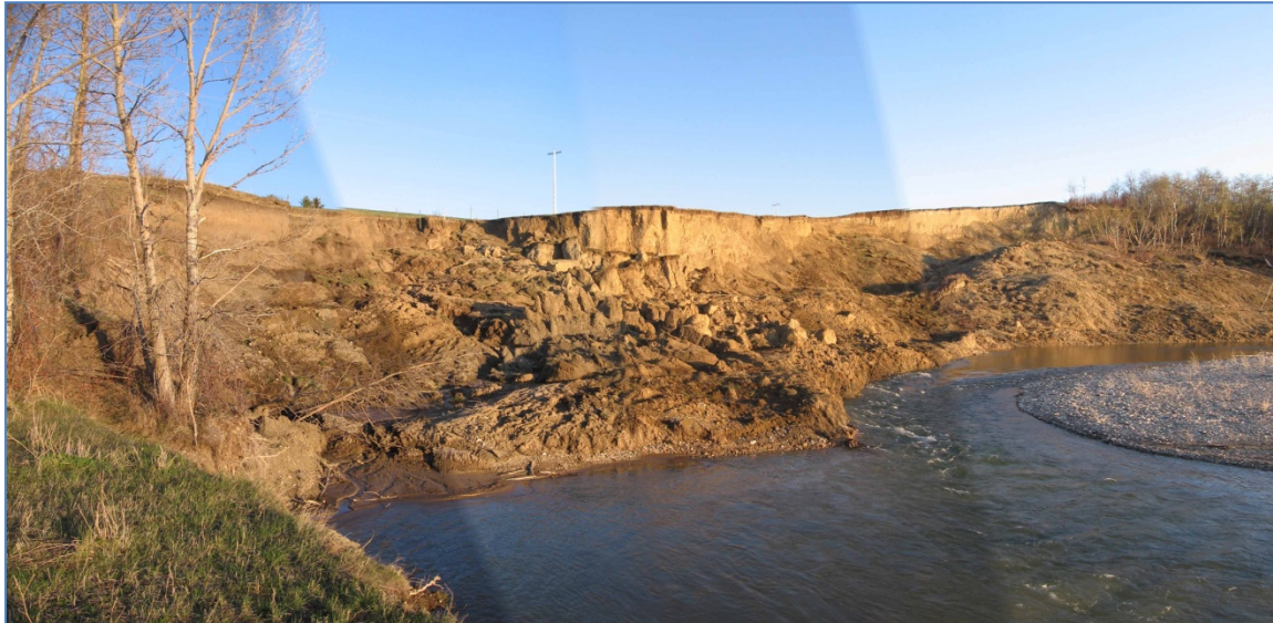
Photo S36-1 (May 2010) – top – Facing southwest and upstream towards the slide area.
