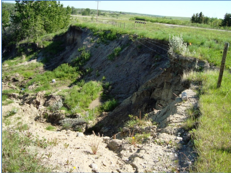
Photo S36-3 (June 2011) Facing northwest towards the main encroachment area with the 2010 regrading and soil nail repair. The landslide does not appear to have retrogressed closer to the road since the June 2010 inspection. The soil nail repair was in good condition.
