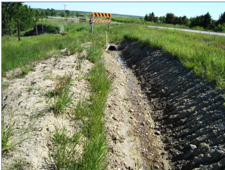
Photo S36-4 (June 2011) Facing north at the main encroachment area and the temporary pipe that has been installed to convey ditch flow across the headscarp area to an armoured outlet north of the site. The ditch and pipe were working effectively.
