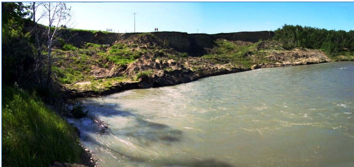
Photo S36-2 (June 2011) – bottom – Photo of the slide area taken from the same location as Photo S36-1. The slide mass that encroached into the river in early 2010 has been largely removed by river erosion. The blocky appearance of the slide mass has become somewhat subdued by erosion and some natural revegetation has taken hold. It appears that the landslide has not moved significantly since May 2010.
