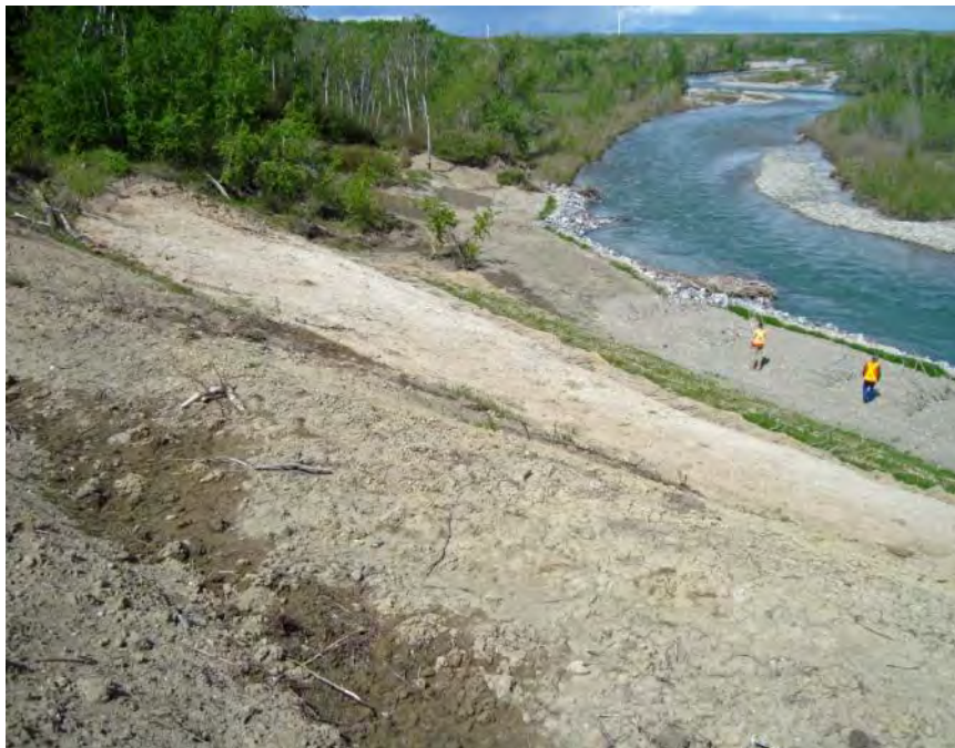
Photo S36-10 - (May 2013) Looking downslope towards the southwest from mid-slope at the area containing bio-engineering repairs.
