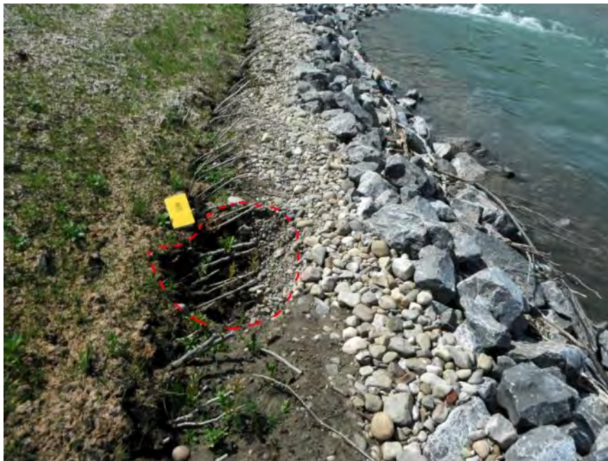
Photo S36-12 - (May 2013) Standing at the east edge of the river bank at the north end of the site. An erosion / settlement area was noted between the rip-rap and willow plantings at the toe of the slope.
