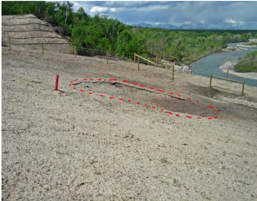
Photo S36-9 - (May 2013) Standing on a bench upslope of the access road within the main slide area looking towards the west at a settlement area around an old piezometer installation. The extent of the settlement is outlined in red.
