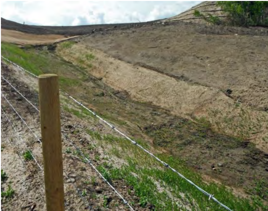
Photo S36-7 - (May 2013) Looking upslope towards the southeast at the south collection ditch. The ditch was wet and vegetation growth was visible.
