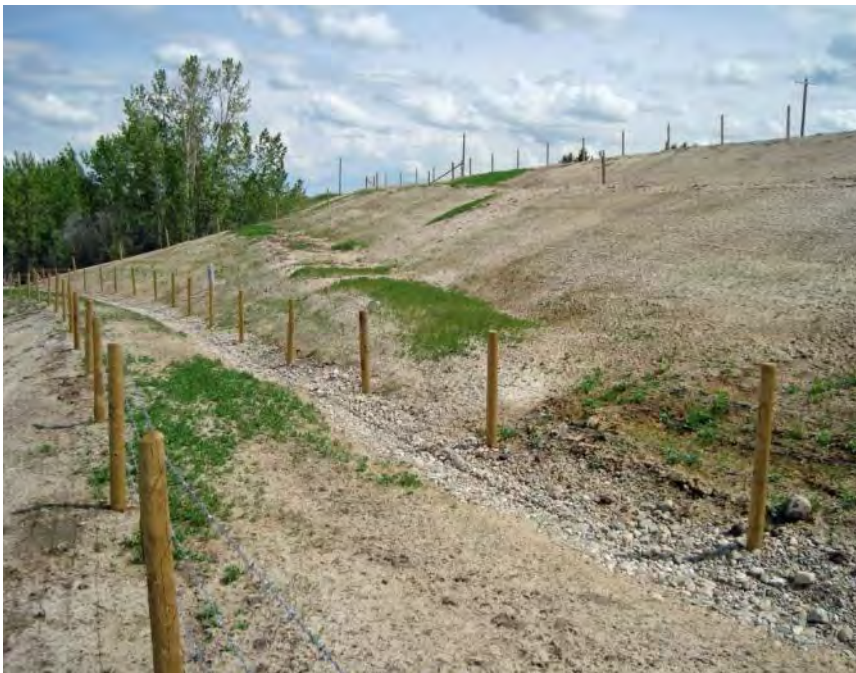
Photo S36-8 - (May 2013) Standing at mid-slope within the main slide area looking towards the north at the fenced access road and upper slope benches.
