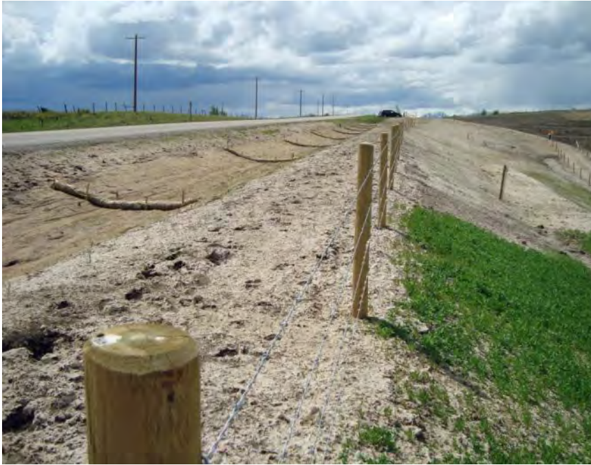
Photo S36-13 - (May 2013) Standing at the fenceline along the slope crest within the main slide area looking south across the west highway ditch and upper bench face.
