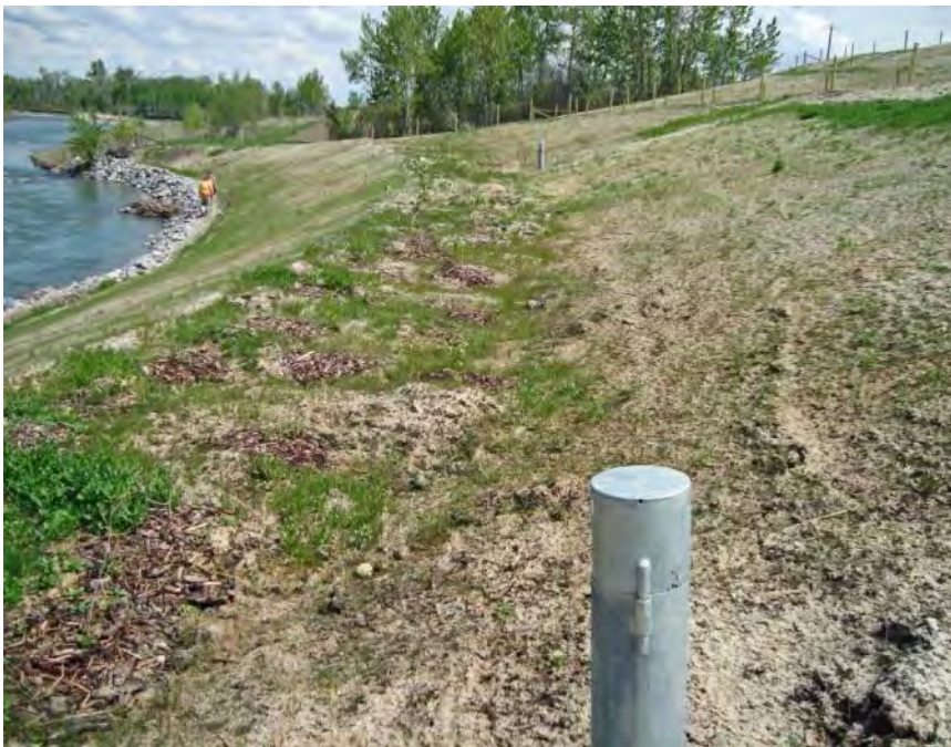
Photo S36-6 - (May 2013) Standing at the southern edge of the main slide area looking towards the north across the lowermost bench.
