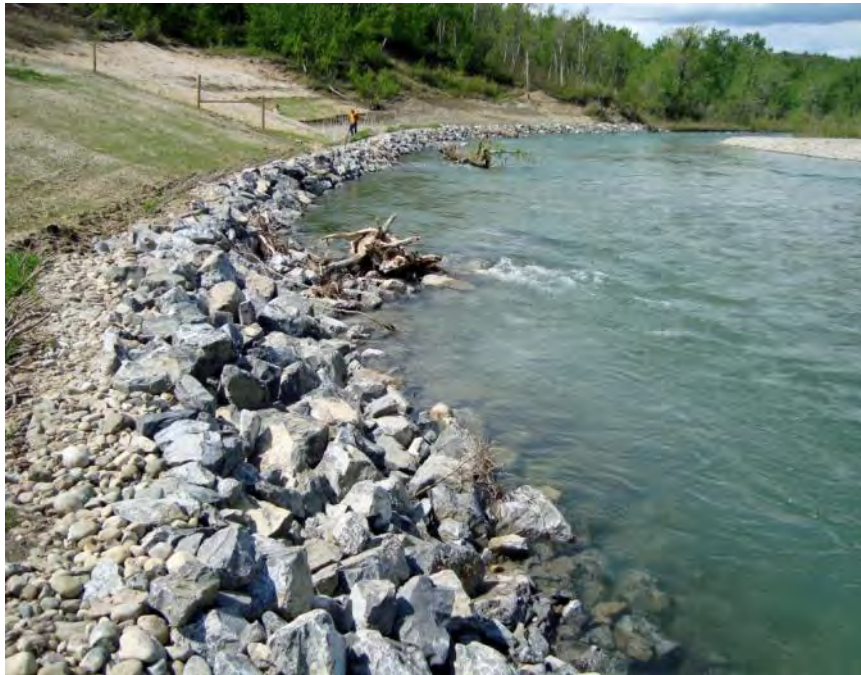
Photo S36-11 - (May 2013) Standing at the east edge of the river bank, at approximately the center of the site, looking towards the south at the LPSTP and vanes. Wood debris had collected in the vanes.
