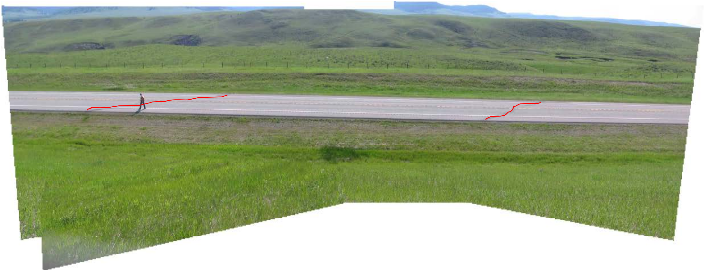
Photograph 5 – Stitched panoramic of Km 15.8 Site taken from the slope above the site. The cracks in the road surface are marked for clarity.
