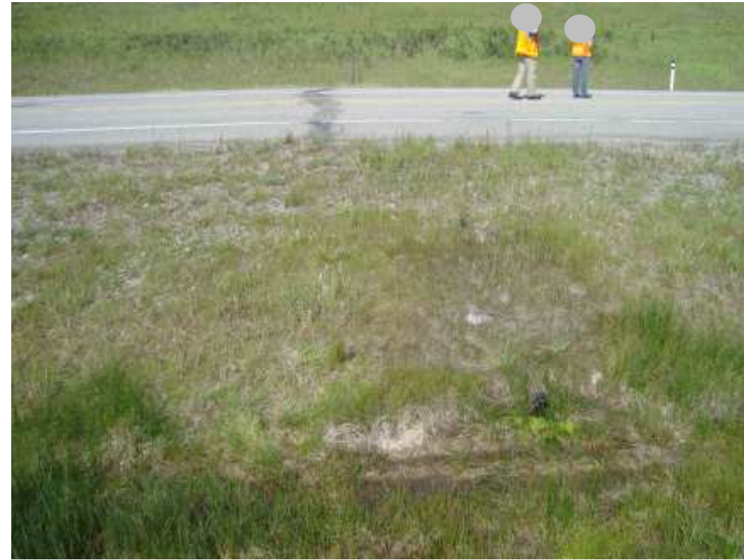
Photograph 2 – Top Left – Cracks in the road surface at Km 15.8 Site.
