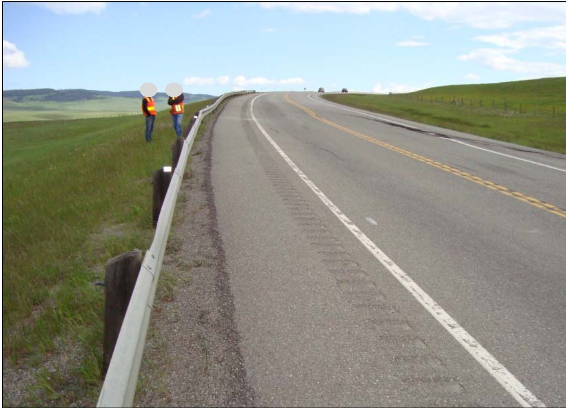
Photo S38-3 - June 2011 Facing southbound across the slide area.
