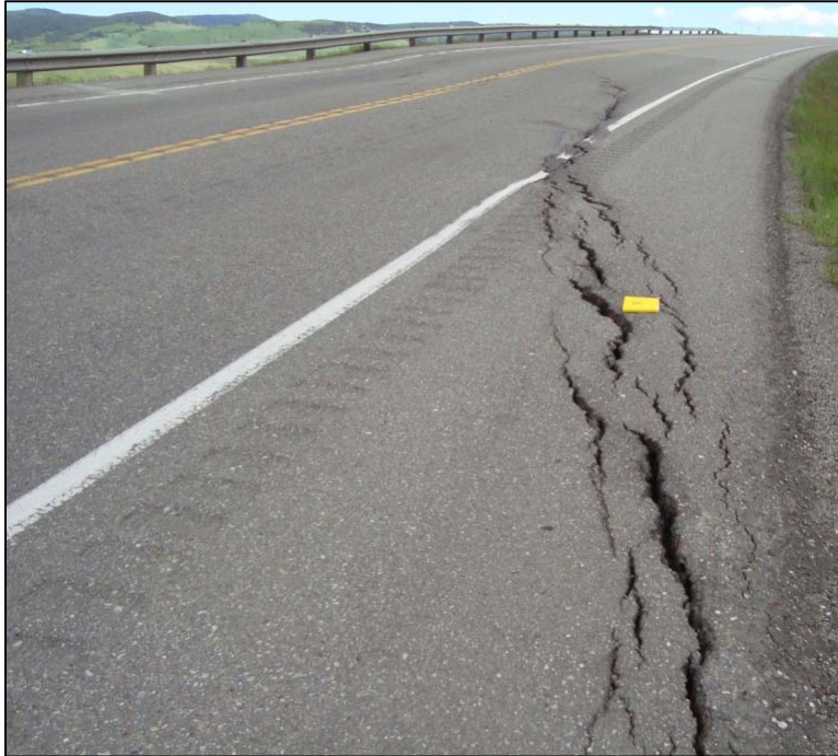
Photo S38-1 - June 2011 Facing southbound across the cracks in the road surface. Note the settlement visible in the upper left corner of the photo near the guard rail.
