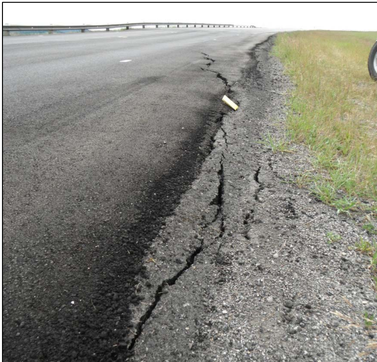
Photo S38-2 - July 2011 Photo taken from the same location as Photo S38-1, approximately one month later. The road has been paved within the last month, with cracks forming through the overlay.
