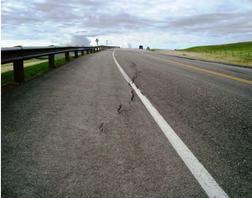
Photo S38-1 (May 2013) Facing south from the east side of the highway. Minor cracking and settlement was visible through the previous overlay.
