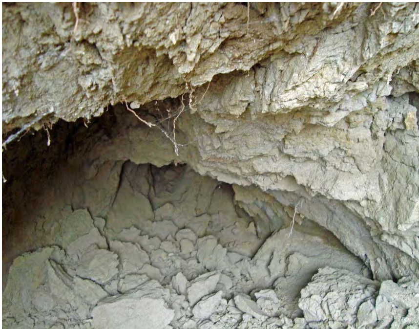
Photo S40-3 – June 22, 2012 An example of a sub-surface erosion tunnel connected to one of the holes discovered at ground surface. The soils in this area were highly susceptible to erosion.
