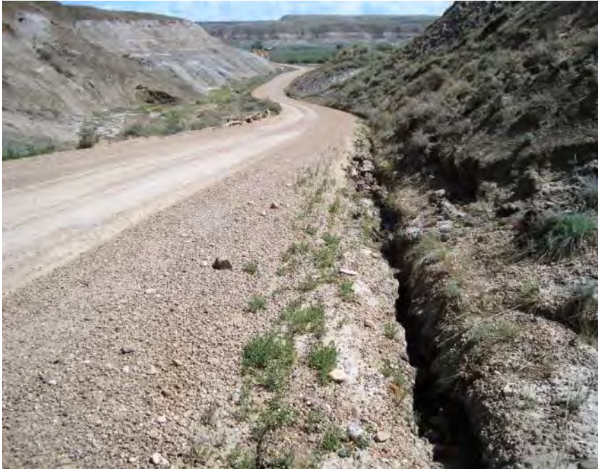
Photo S40-3 – May 2013 Standing on the southeast road shoulder looking towards the east at the south ditch erosion.
