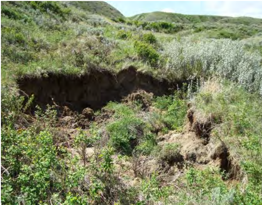
Photo S40-1 – May 2013 Standing south of the highway looking at the apparent recent collapse of a sinkhole observed around the area marked by WPT 60 on the site plan.
