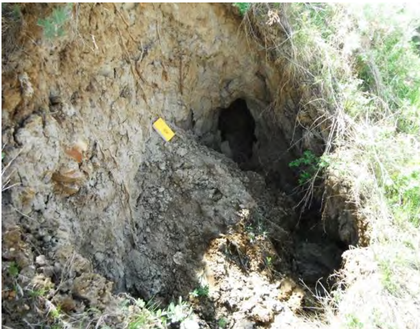
Photo S40-2 – May 2013 Standing at the north highway edge looking towards a collapsed sinkhole that has eroded a vertical face up to the road. A tunnel appears to be connected that runs beneath the highway located at WPT 105.
