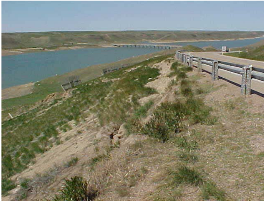
Photo 1 – View of downslope edge of the road showing the proximity of the landslide scarp to the guardrail (May 2002).
