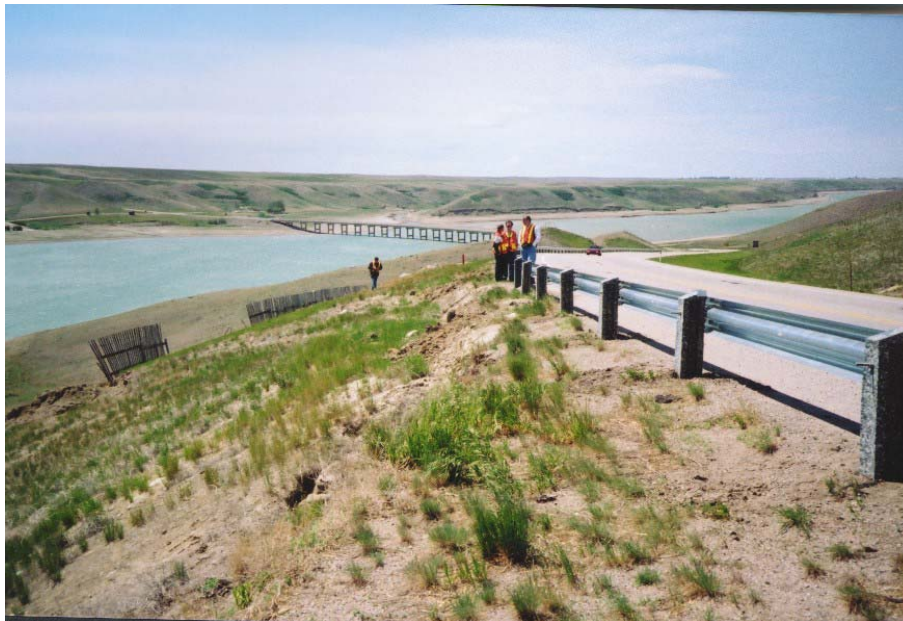
Photo 2 – Downslope edge of road as seen during the May 2001 inspection.
