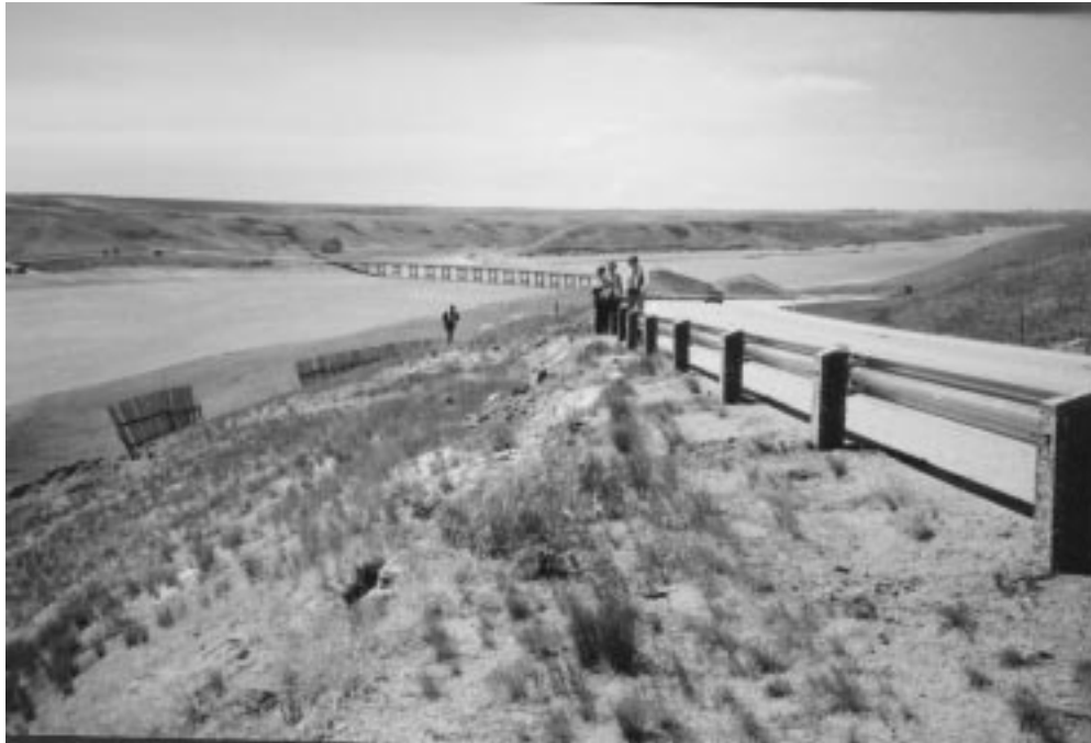
Photo 1 – View of downslope edge of the road above slide area (2001). Note newly-installed guardrail and slide scarp visible downslope of road.
