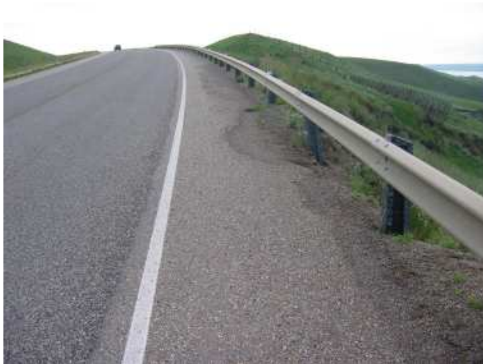
Photo S5-2 (lower left) – June 2005 – facing east along eastbound lane. Note the settlement in the shoulder next to the guardrail.
