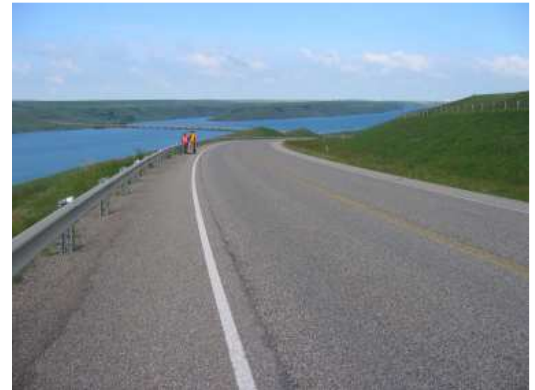
Photo S5-5 (right) – facing west along road. No new cracking visible since the last annual inspection.
