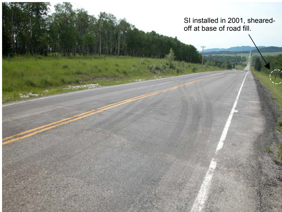
Photo 3 (lower left) Another view of the cracking in the southbound lane, north end of the site.
