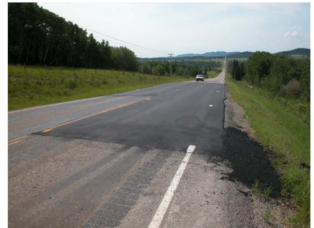
Photo 4 (lower right) Facing south across the recently repaved southern cracking and settlement area at this site. The instruments that were installed in the fall of 2002 in this area have measured ongoing slope movement towards the southwest. The rate of slope movement has been moderate, and cracking of the road surface has resulted. This repaving has “reset” the road surface with respect to cracking, but unfortunately prevented any observations the magnitude and extent of additional cracking since the previous site inspection in May 2002.
