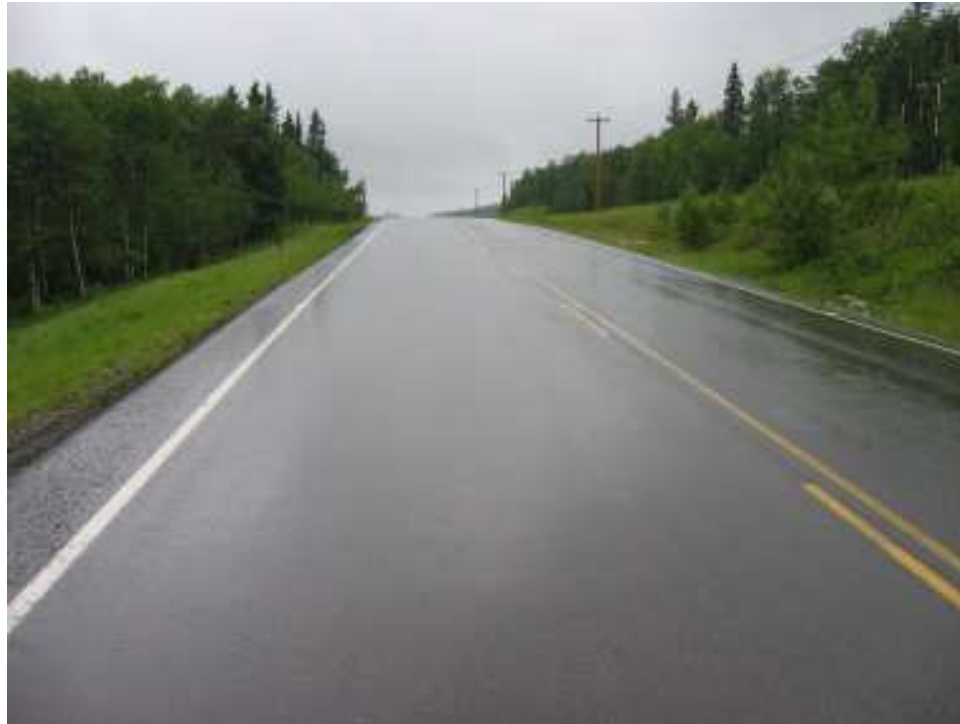
Photo S8-1 (upper left) – June 2005 – facing north across the northern area of the site. No significant cracking or settlement was noted.
