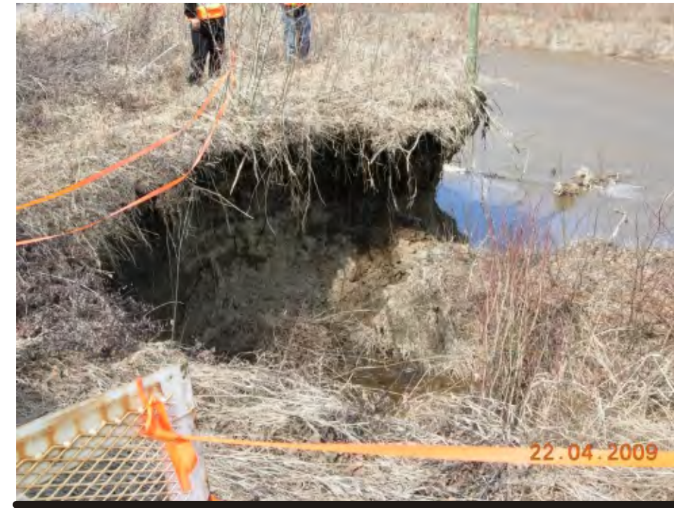
Photo 2 Looking north at scour location
