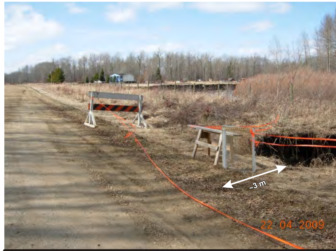
Photo 4 Looking northwest at scour location - Crest of scour within 3 m of edge of roadway - Area barricaded and demarcated to notify motorists of reduced setback distance and to minimize public access into area
