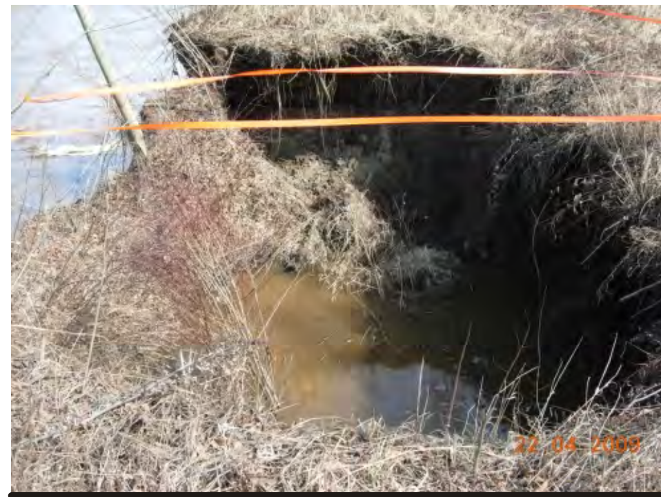
Photo 1 Looking east at river bank scour location
