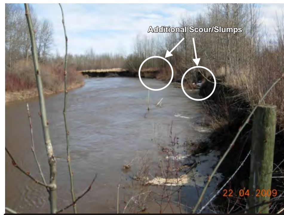
Photo 3 Looking east (downstream) at additional slumps/scours along south bank of Driftpile River (right hand side of photo)
