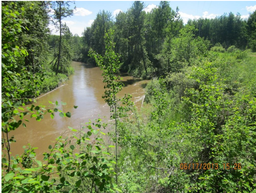
Photo 1: Location where Driftpile River bank is encroaching on local road looking south west
