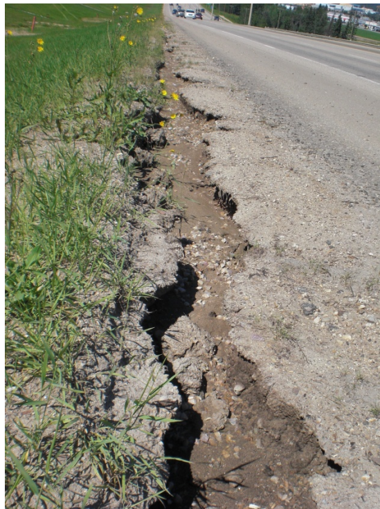
Photo 4: Erosion along outside shoulder of eastbound lanes.
