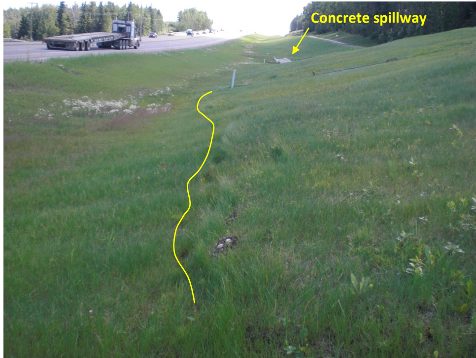
Photo 3: Toe bulge on south side of highway, facing east.
